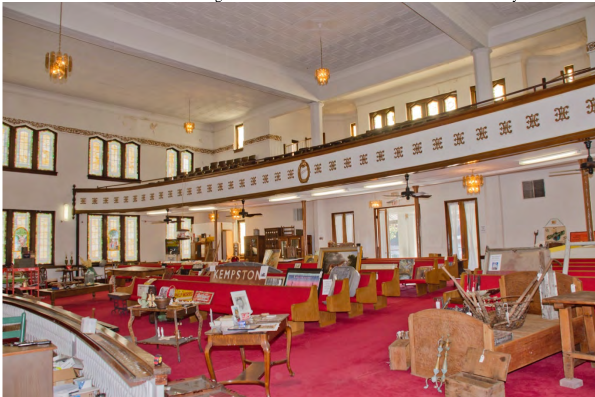
Photo 11: First floor interior showing structural beams and interior ornament. Sanctuary. View southeast.
