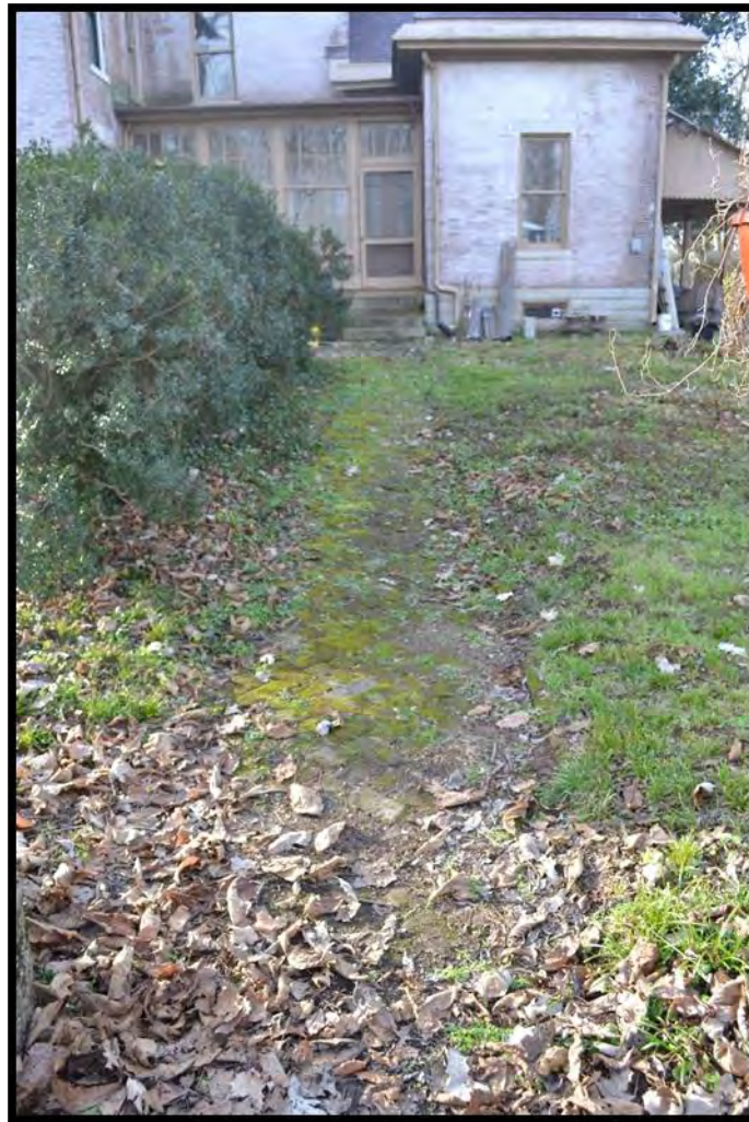
Figure 6. Brick walkway leading to east elevation porch, looking west toward interior service spaces. (Photo 0002).
