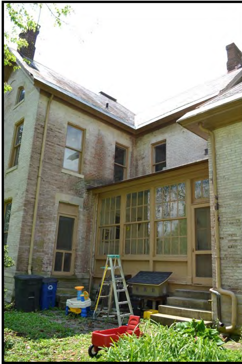
Figure 15. The projecting gable has a rear north-facing elevation with a door and several second story windows, looking southwest. (Photo 0010).
