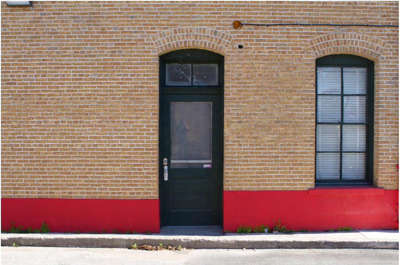
Photo No. 8. Detail view of the door to the original fire marshal's office, and window, both with brick arches. View facing southwest.
