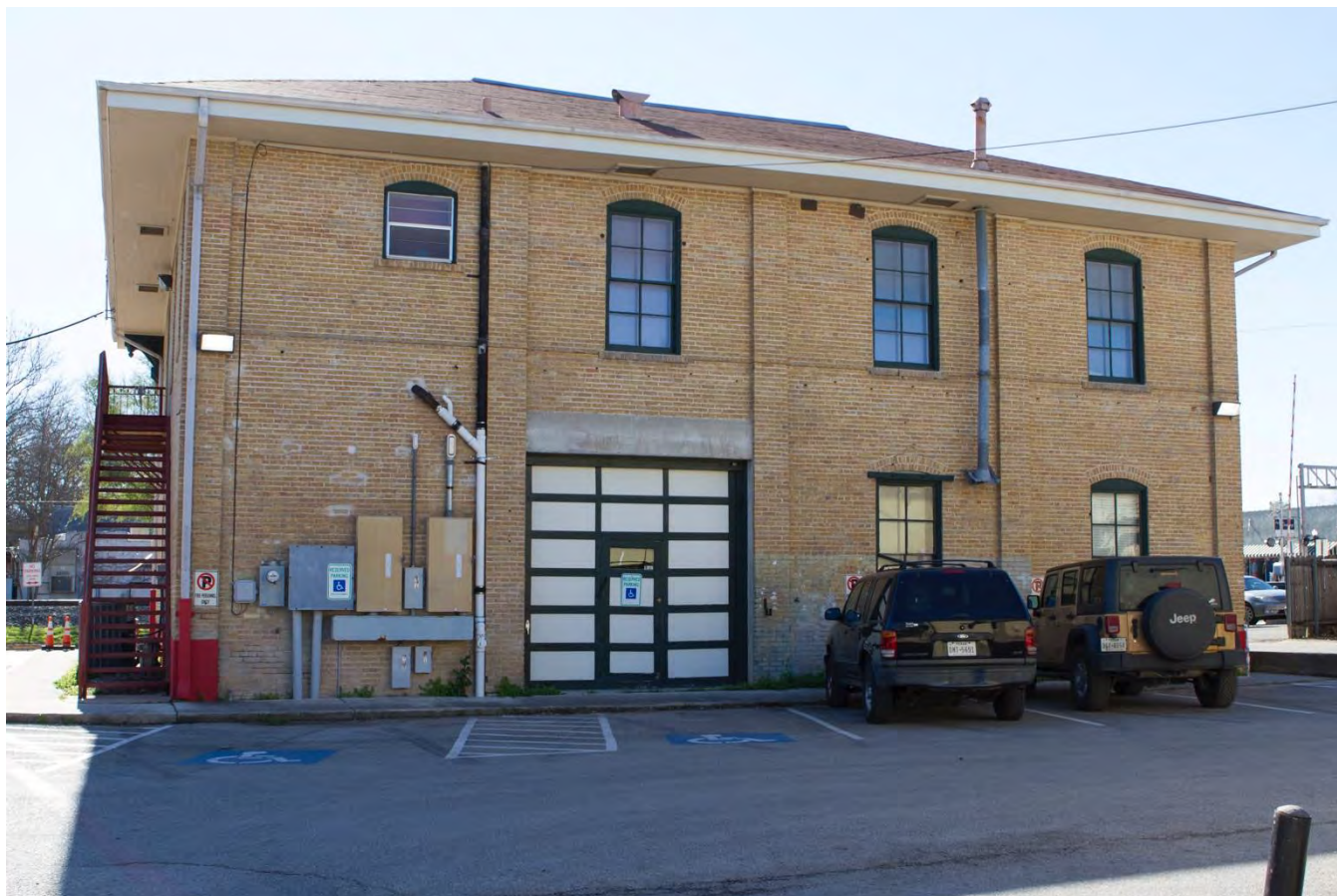
Photo No. 4. View of the Central Fire Station, view facing southwest. The remnants of an awning, added sometime before 1980 and since removed, are evident on this façade below the second story windows.
