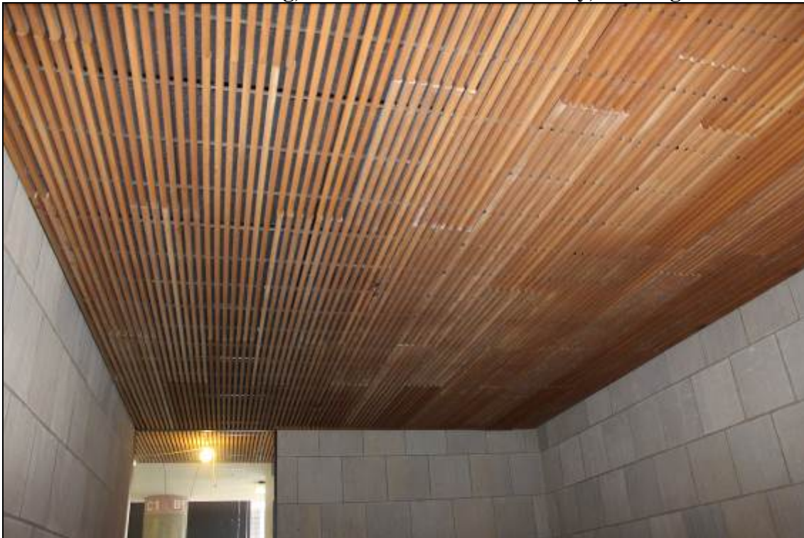
Photo 15: FHLBB Building, Slot Wood Ceiling in High-Bay Portion of East Lobby, Looking North
