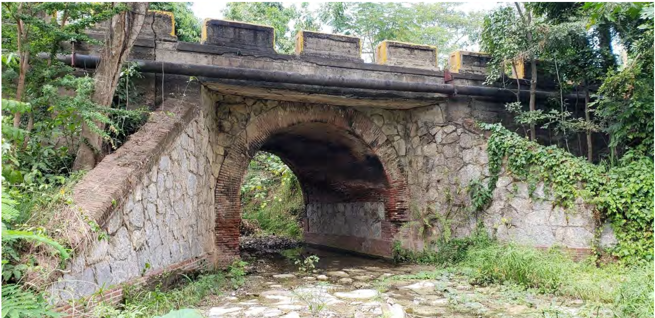
Another hidden treasure from the 19 th century, this brick and stone structure, is in PR-14, Km. 19.7 in Juana Díaz. Because of its size, over four meters in span, using 19 th century standards, the structure could be considered a pontón .
