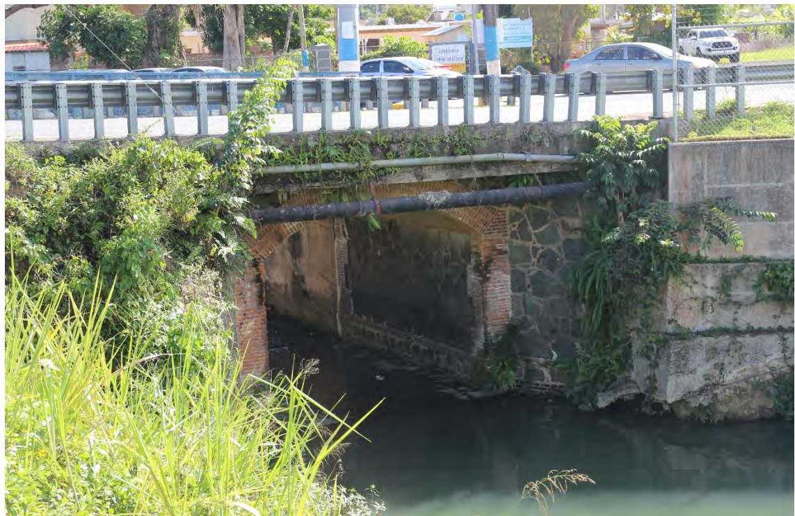
Two pontones in Aibonito. The one at the top is in PR-14, Km. 48.3. The one at the bottom is in PR-14, Km. 51.1.
