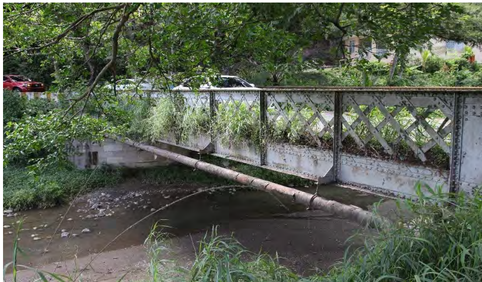
Figure 40. Above, detail of the Raimundo Camprubí's 1874 drawing for the bridge over Río Descalabrado. Below, a partial view of the structure, 2018. 115
