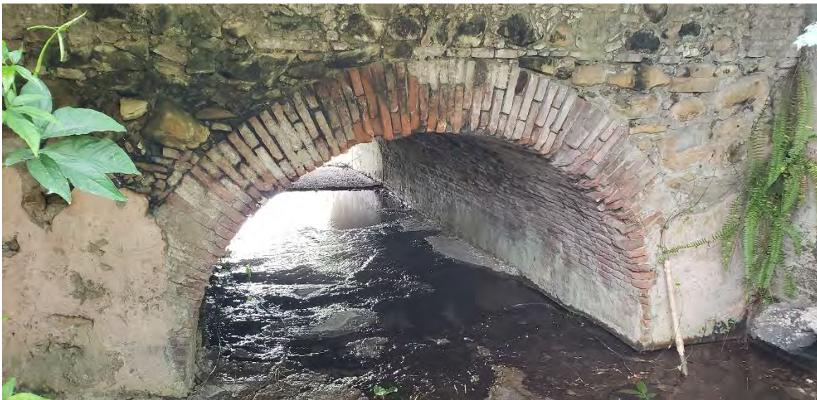
A brick, masonry and stone alcantarilla at PR-14, Km. 11.5 in Juana Díaz.
