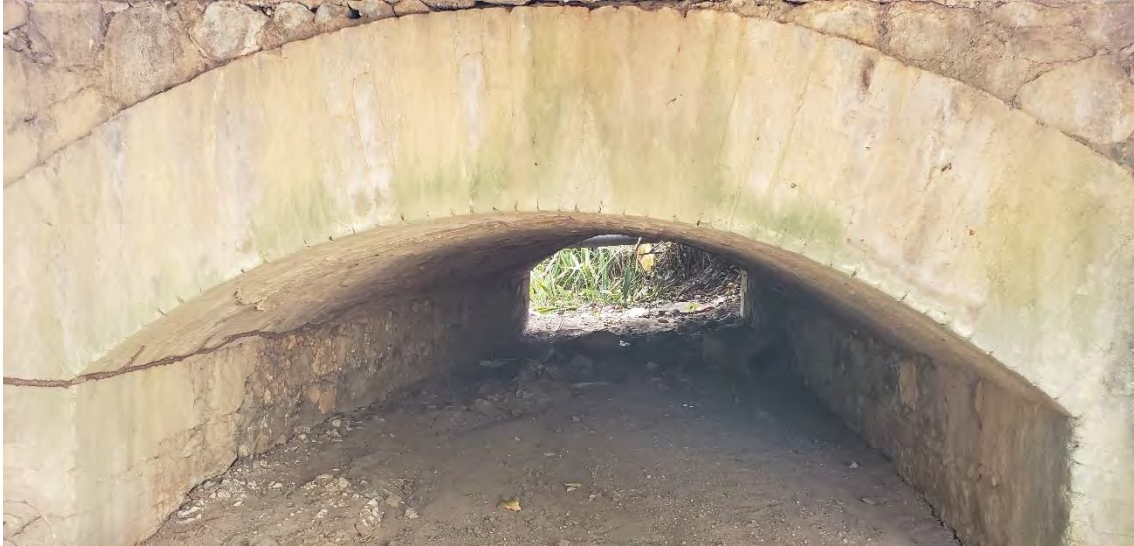
A brick, masonry and stone alcantarilla at PR-14, Km. 18.9 in Juana Díaz.
