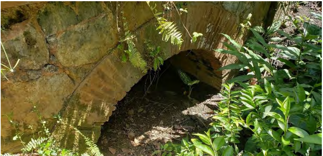
PR-1, Km. 43, Caguas. The neighbors near this alcantarilla recalled that this tajea is just as high as the one shown in the next page, but sediment has built-up through the years. Both structures are just one hundred (100) meters apart.
