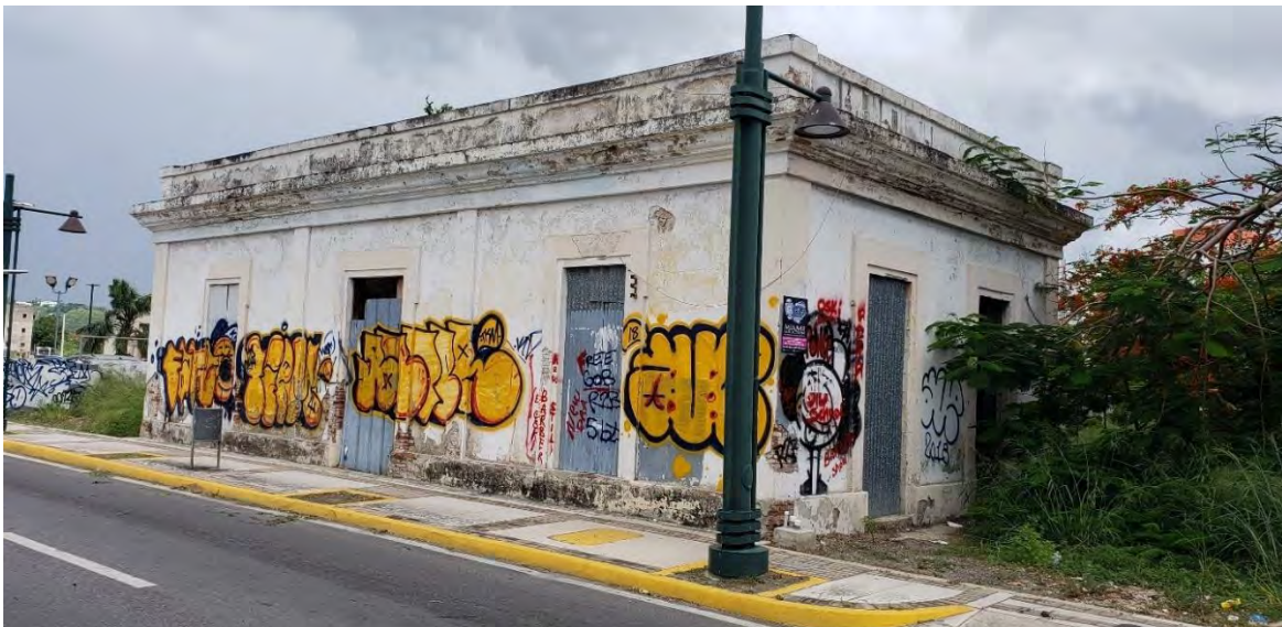
Casilla #16. Located on PR-14, km 3.5, in the municipality of Ponce. Built in 1886, currently abandoned, the building was used by DTOP well into the 1980s.
