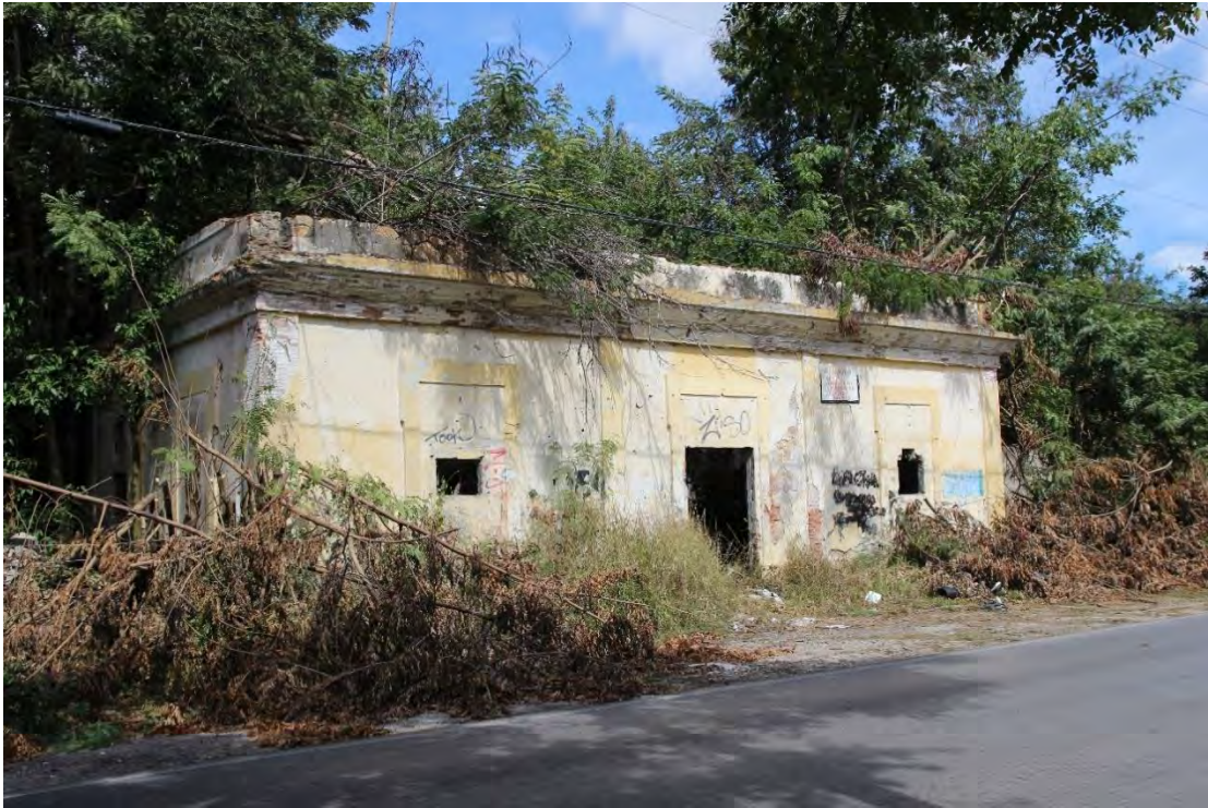
Casilla #15. Located on PR-14, km. 10.3 in Juana Díaz. Built in 1886, this abandoned casilla was used by DTOP until the 1950s. It served as a warehouse for an agricultural firm and later became the well-known brothel El Reloj .
