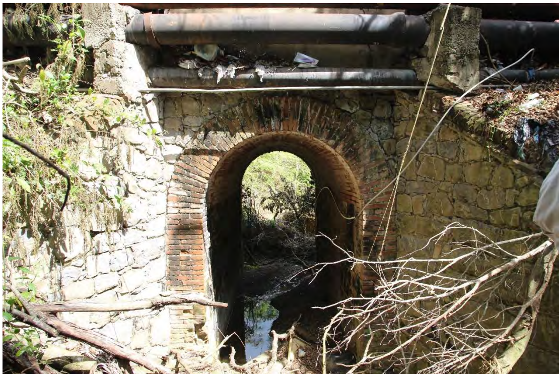
On the picture above, PRSHPO staff searching for the best route to access the tajera shown below, located at PR-14, Km. 35.4 in Coamo.
