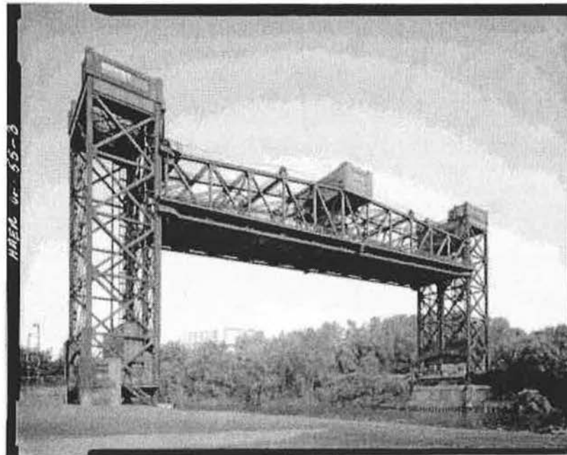
Figures 20 and 21. Columbus Road Lift Bridge in lowered and raised position. (source: HAER, photos by Randal Gooden)
