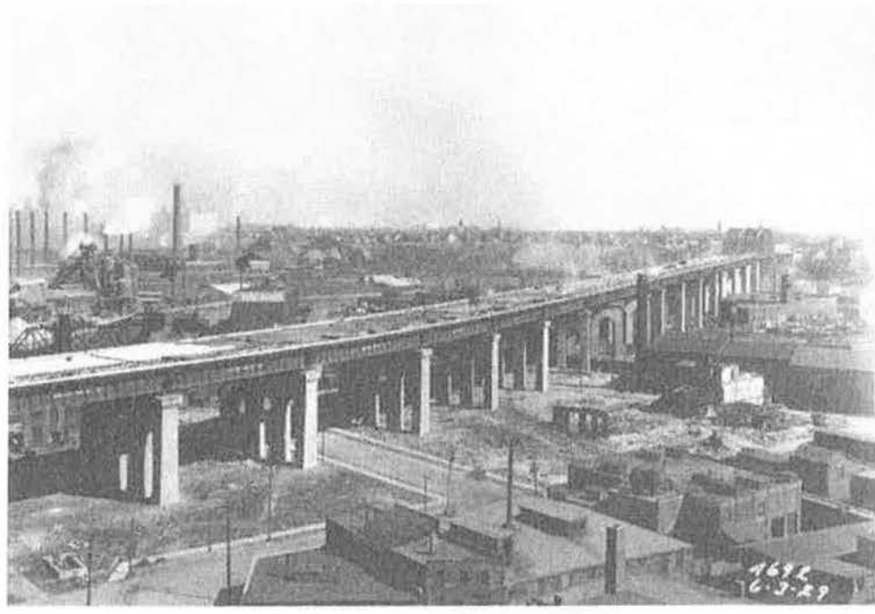
Figures 23 and 24. Construction photos of the Cleveland Terminal Viaduct (Cuyahoga Valley Viaduct). The river span is above and the lower photo is an image of it crossing through the proposed district. The district has always had a lot of empty land, as evidenced in this photo from the 1920s. The piers for this bridge, as well as the Detroit-Superior High Level Bridge, extend across the district with undeveloped land beneath them.
