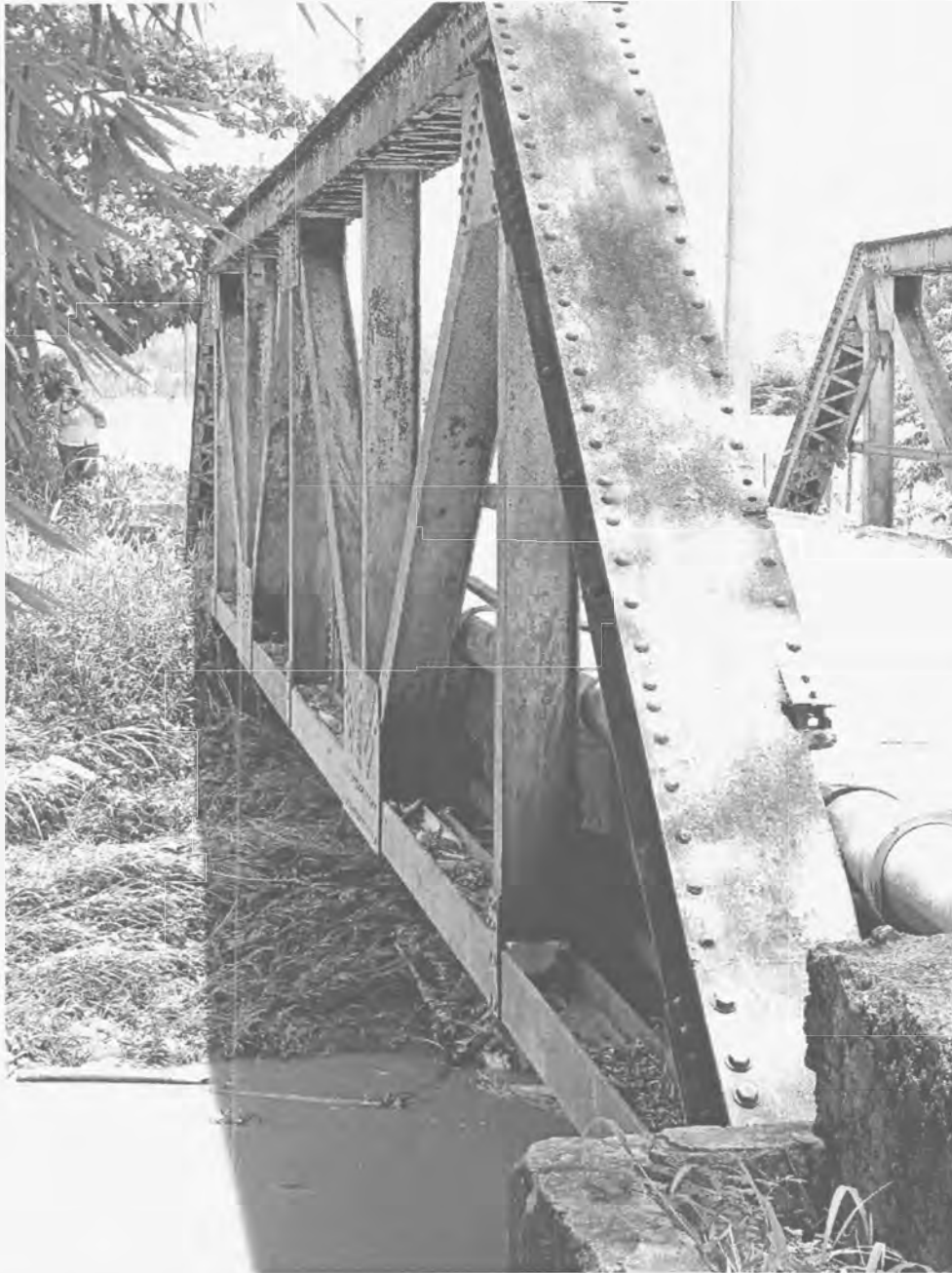
Bridge #1142 – Close up of endpost and lower chord of the eastern side as seen from the bridge’s northern end. Taken by José Marull, PRSHPO, on May 11, 2010.
