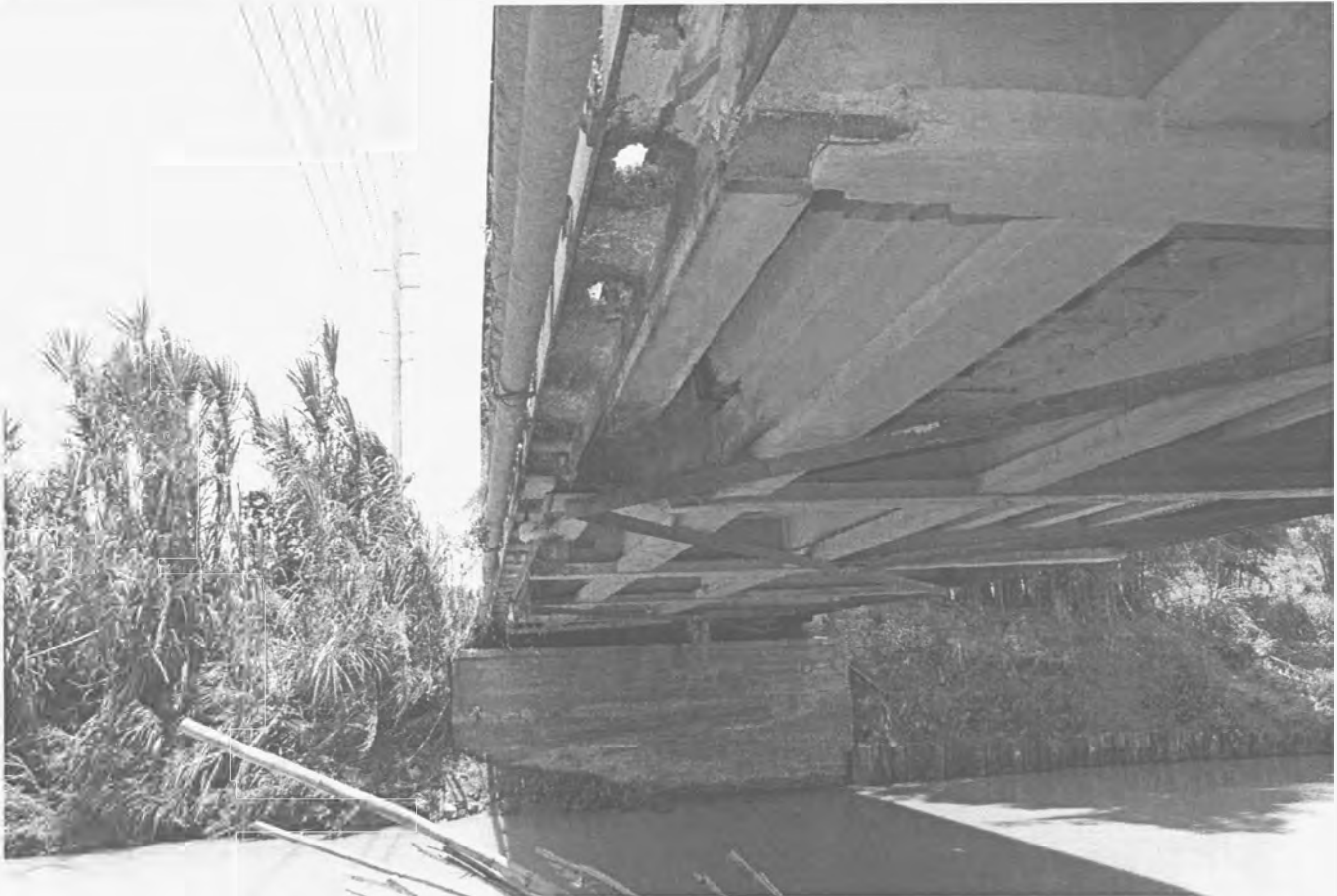
Bridge 1142 – View of Culebrina River, southern abutment, bridge stringers, bottom lateral bracing and floor beam. Taken from beneath the bridge by José Marull, PRSHPO, on May 11, 2010.
