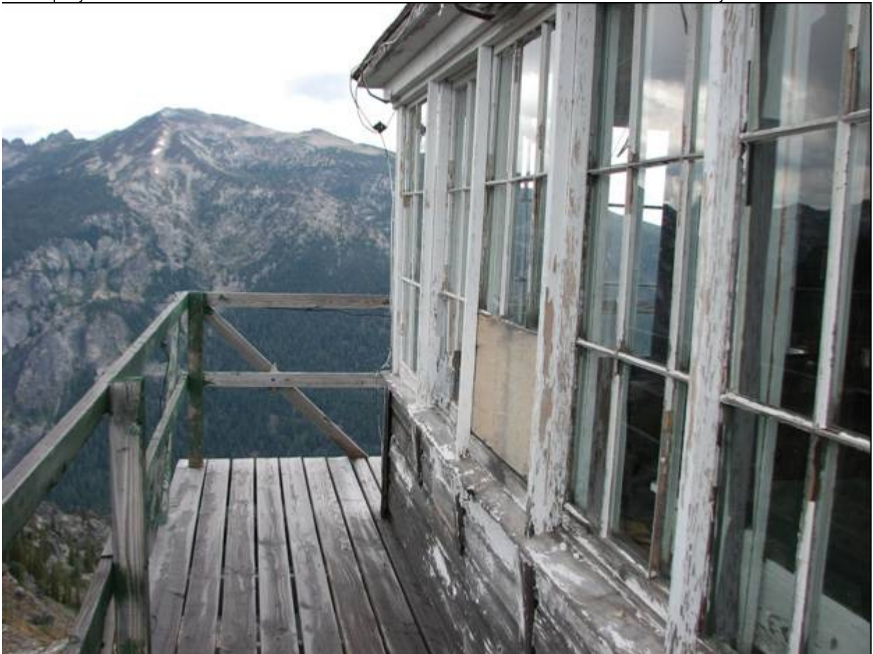
MT_RavalliCounty_BoulderPointLookout_0003. Looking north along the west side of the catwalk over the Boulder Creek Drainage to Trapper Peak.
