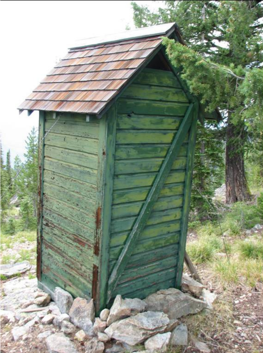
MT_RavalliCounty_BoulderPointLookout_0007. Looking southwest to the east and north (rear) wall of the outhouse
