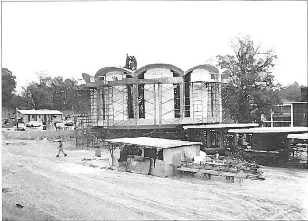
Figure 12. Monroe Drive branch building under construction, Atlanta, Georgia, November 13, 1961. LBCB108-060b, Lane Brothers Commercial Photographers Photographic Collection, 1920-1976. Photographic Collection, Special Collections and Archives, Georgia State University Library.
