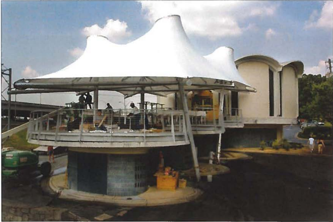
Figure 18. Workers add finishing touches to Piebar, former Trust Company Bank building during renovations to convert it to a restaurant, July 2005. Photo from the Atlanta Journal-Constitution, by Joey Ivanescu / AJC staff.
