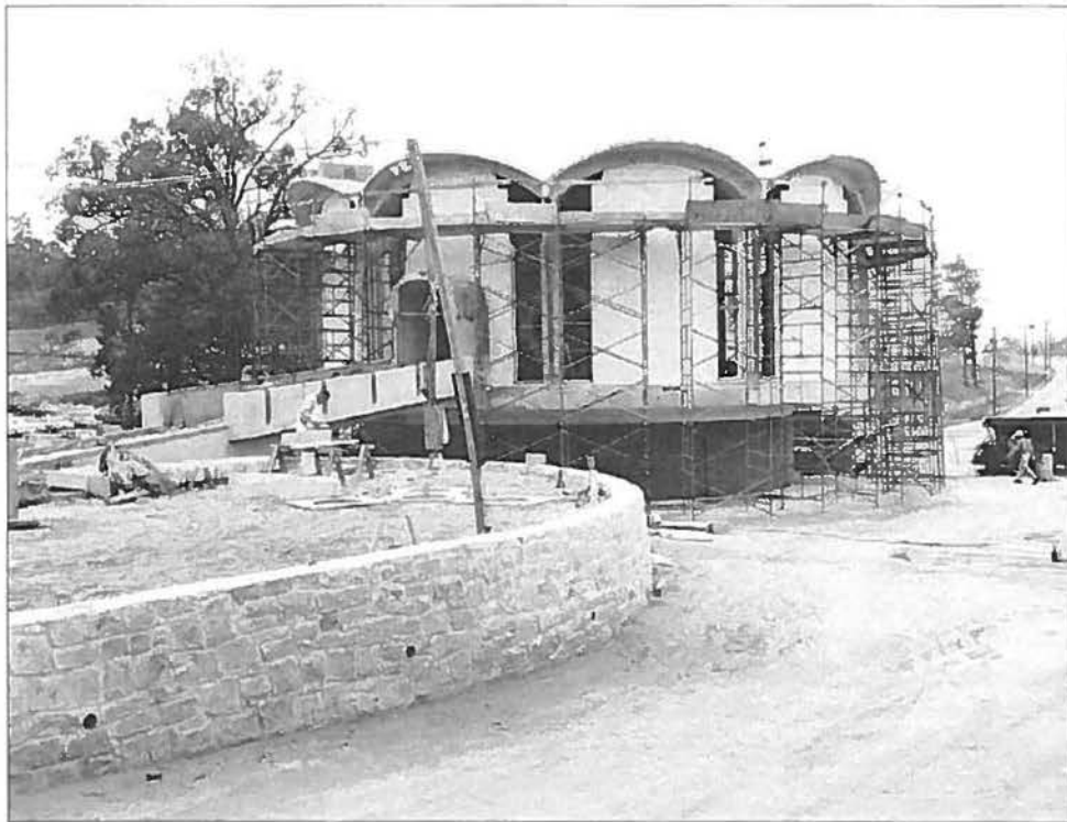
Figure 11. Monroe Drive branch building under construction, Atlanta, Georgia, November 13, 1961. LBCB108-060c, Lane Brothers Commercial Photographers Photographic Collection, 1920-1976. Photographic Collection, Special Collections and Archives, Georgia State University Library.
