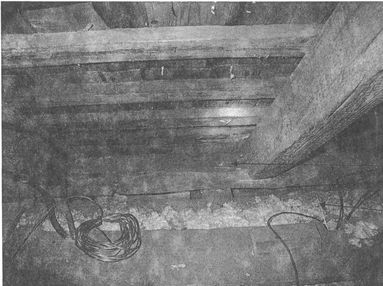
Figure 1: double plate roof framing on the front of the house, view north
