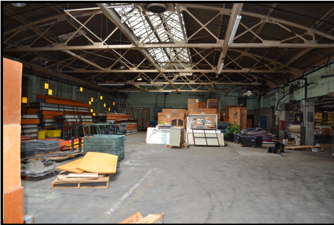
Figure 36. Interior view of circa 1946 addition, looking west. Note the clerestory of skylights and the distinctive metal truss roof support. (Photo 0020).
