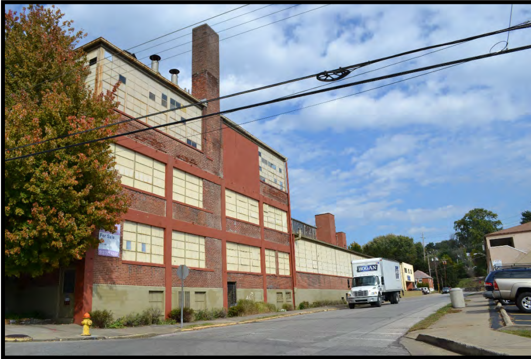
Figure 9. South elevation/Primary facade of Grote Building, looking NE. The 1924 portion of the building is located in the foreground. The one-story circa 1946 addition can be seen in the background. (Photo 0002).
