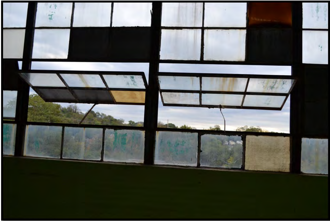
Figure 34. The fourth floor is characterized by bands of metal pivot windows, as seen on the north elevation in the photo above. Photo taken looking northwest. (Photo 025).
