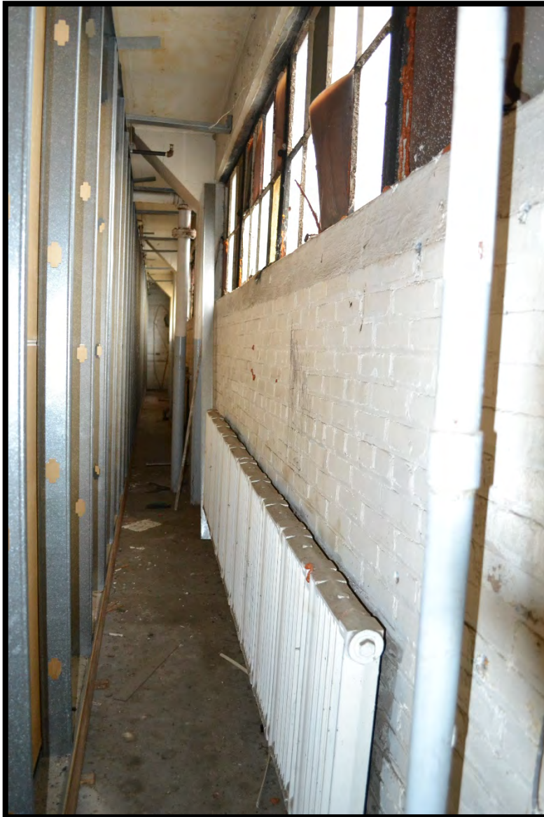
Figure 32. The original brick veneer (and terra cotta block) walls are visible behind the modern partition wall on the 1925/1946 addition's south wall on the second floor. (Photo 0018).
