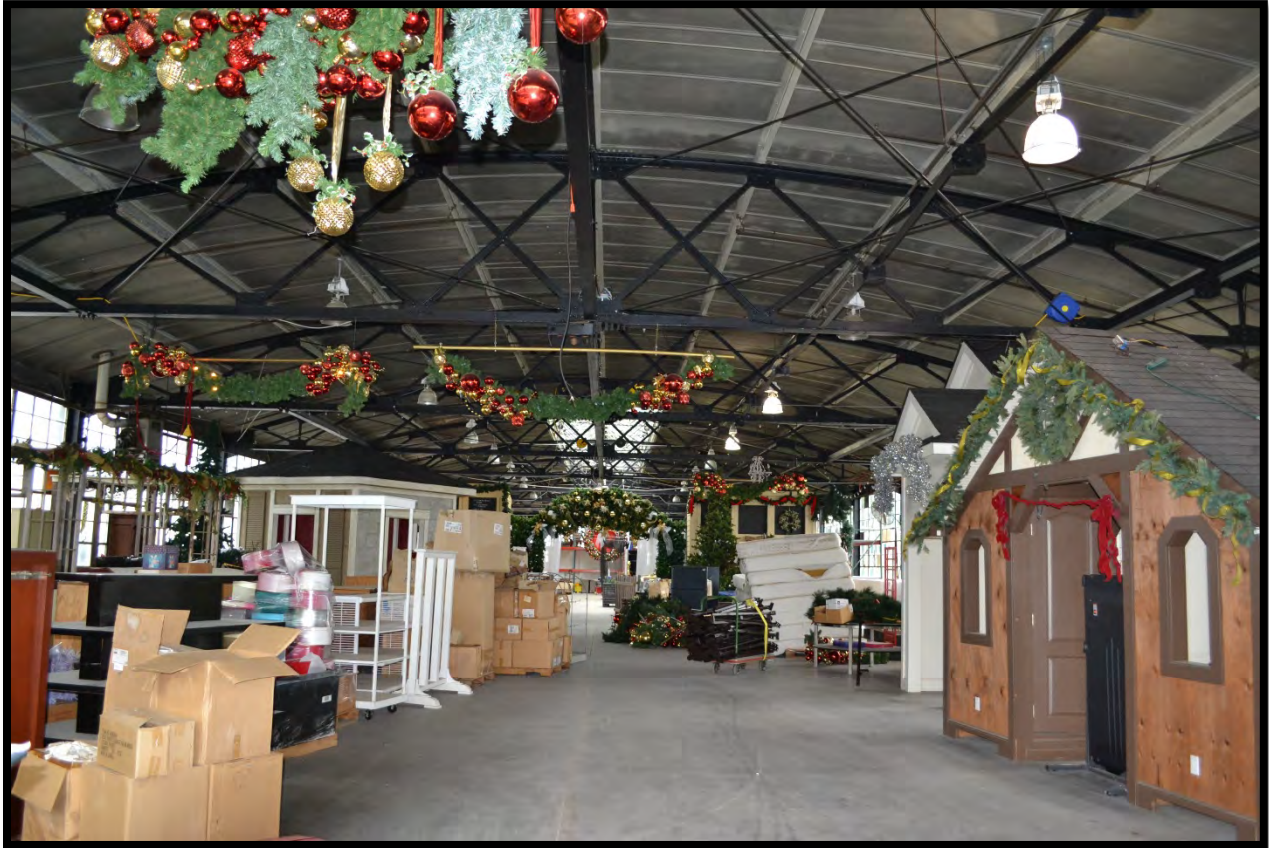
Figure 33. The fourth floor features a barrel vault roof and clerestory of skylights, visible in the background. Photo taken looking west. (Photo 024).
