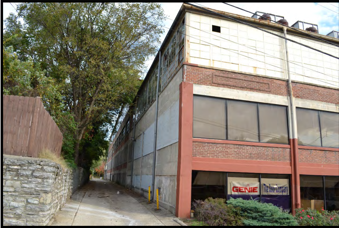
Figure 18. View of rear (north elevation), looking east. The 1924 portion of the building is in the foreground. (Photo 0010).
