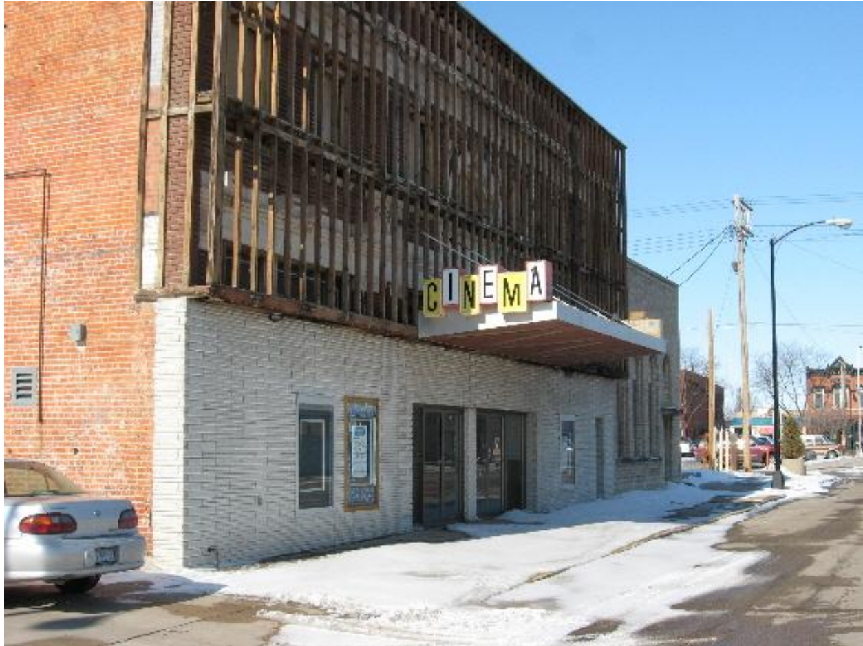
Figure 3. Grand Theater during rehabilitation, March 6, 2008. Photo by LuAnnCarter. Photo used with permission of Norfolk Community Theatre.
