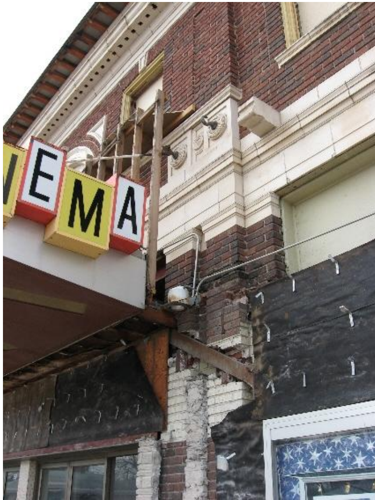
Figure 4. Grand Theater during renovation, March 6, 2008. Photo by LuAnnCarter. Photo used with permission of Norfolk Community Theatre.
