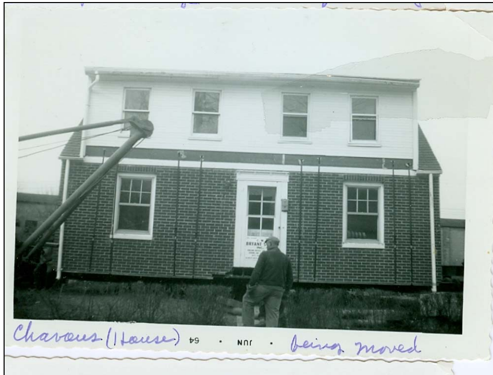
Figure 21: C. W. Bryant and Company moving a house from the Carver Addition
