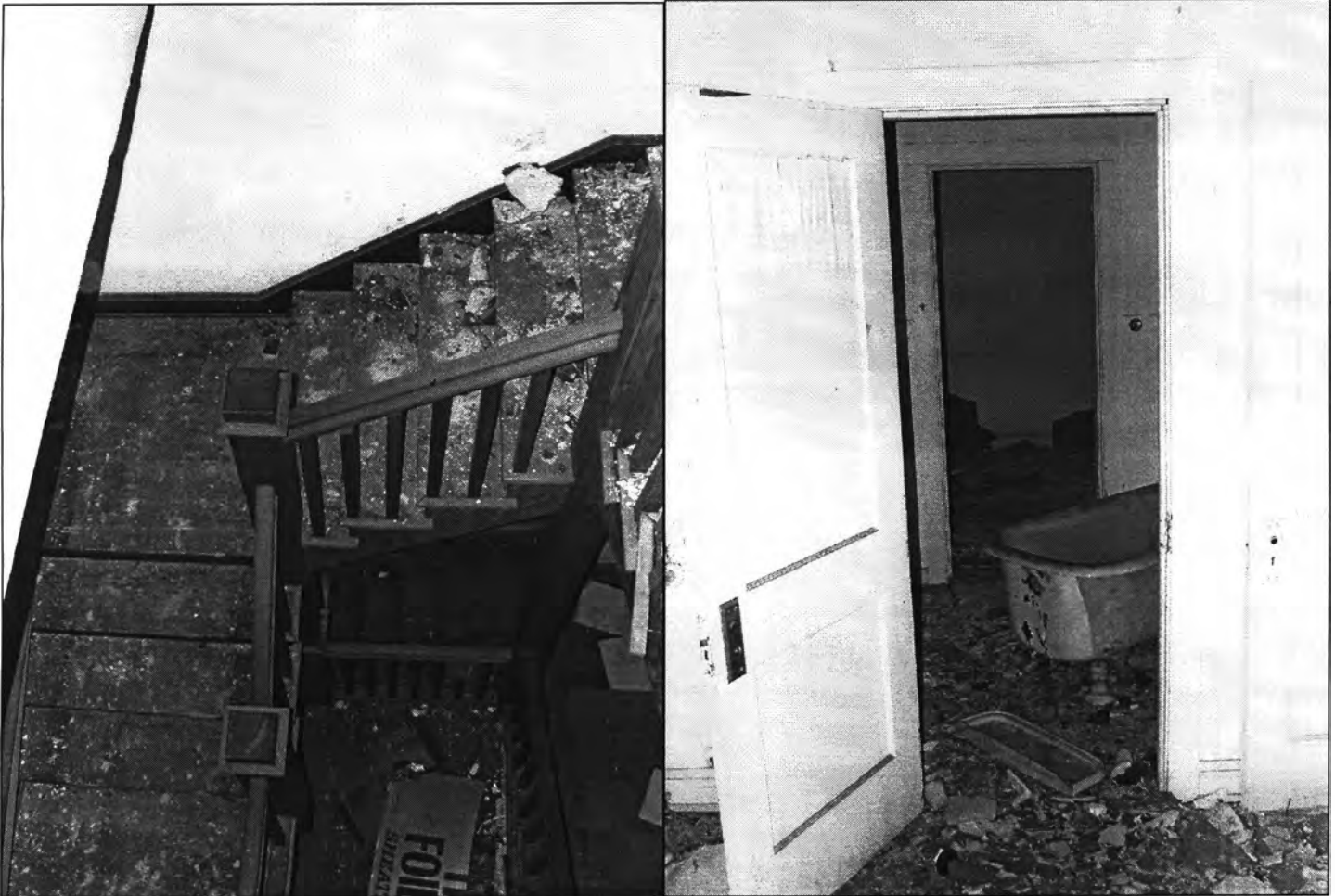
Figure 19: Left, stairway viewed south from third floor, and right, remnant of added bathroom and partition walls, third floor, northwest corner, view west (photos by J. Jacobsen, May 4, 2010)
