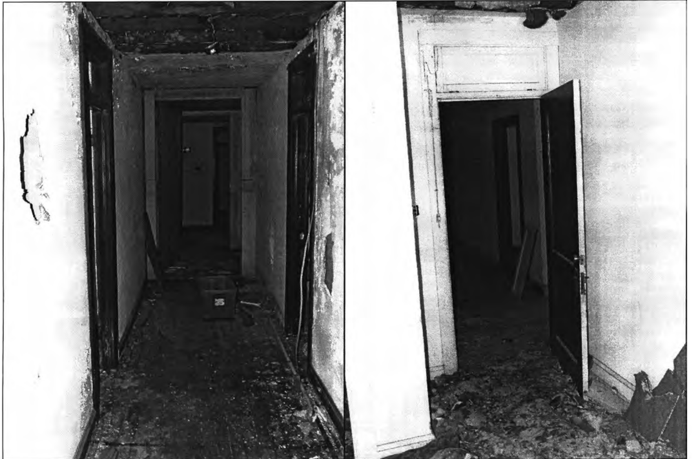
Figure 18: Left, third floor hallway, view east towards stairway (on right side, out of view), and right, third floor north/south hallway viewed from a room in the northeast corner, view southwest (photos by J. Jacobsen, May 4, 2010)
