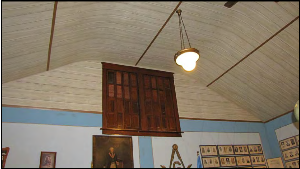
SD_Kingsbury County_Arlington Masonic Temple_0013: Interior detail (main hall looking at north window interior shutters).
