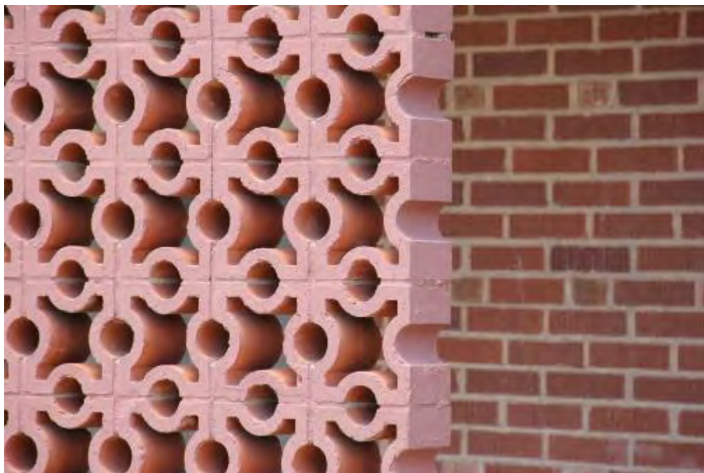
Photograph 10 – Enlarged detail of decorative concrete block screen wall of Apartment Building Type C. Camera facing northeast. (June 29, 2016)
