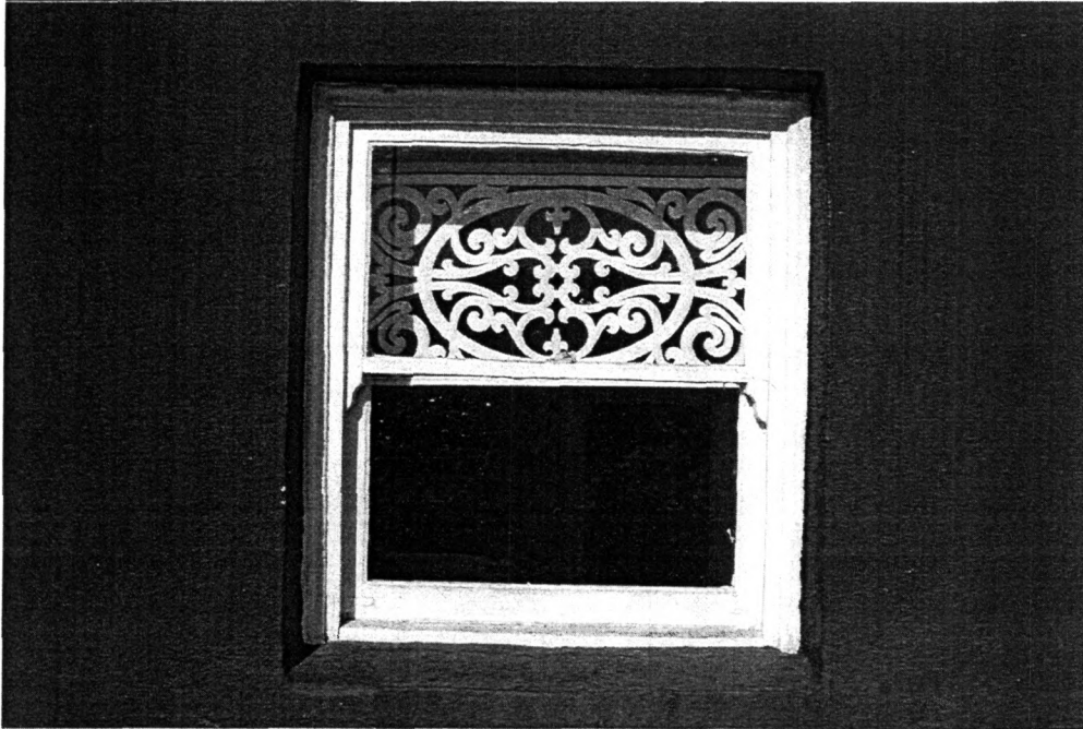
Photo 9 View of a typical basement window in the Meeting House looking west
