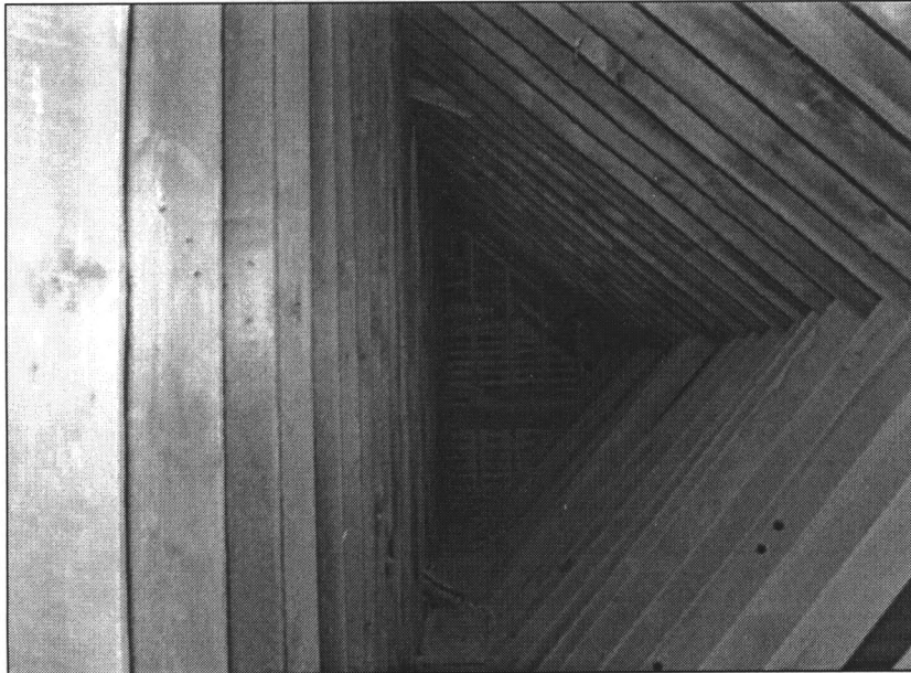
Figure 5: Attic framing, vertical 2x6 posts run down center of plan, angled struts join midway with roof Back or south wall is visible in background, view southward along west side of attic (photo by Floyd Soenksen)
