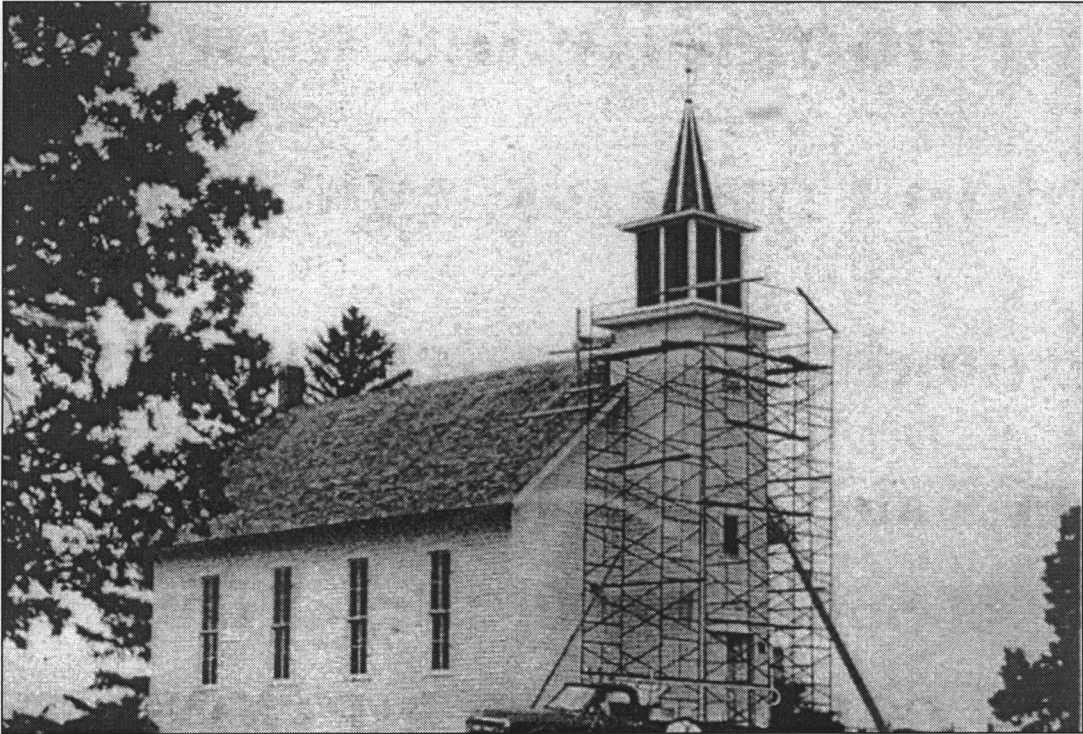
Figure 23: 1977 photo showing the replacement of the spire and base tower, view southwest ( Lost Nation Press , June 29, 1977)
