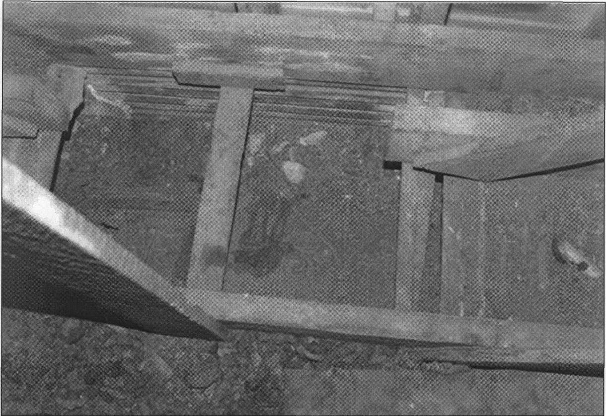
Figure 25: Attic view through former internal chimney passage, showing back side of coved metal roof on south end of sanctuary
