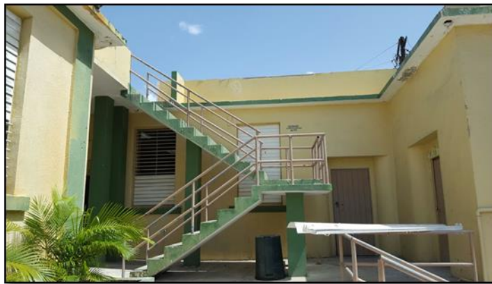
Picture 6: The dog-leg shaped stairway that currently serves as access to the roof.
