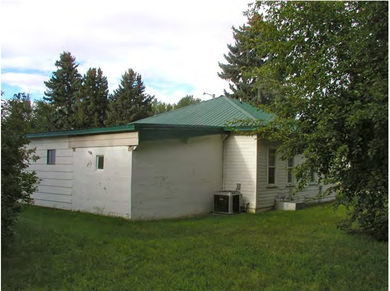
Description and view of camera: North and East elevations, view to southwest Photograph: MT_YellowstoneCounty_HuntleyProject Office_0004
