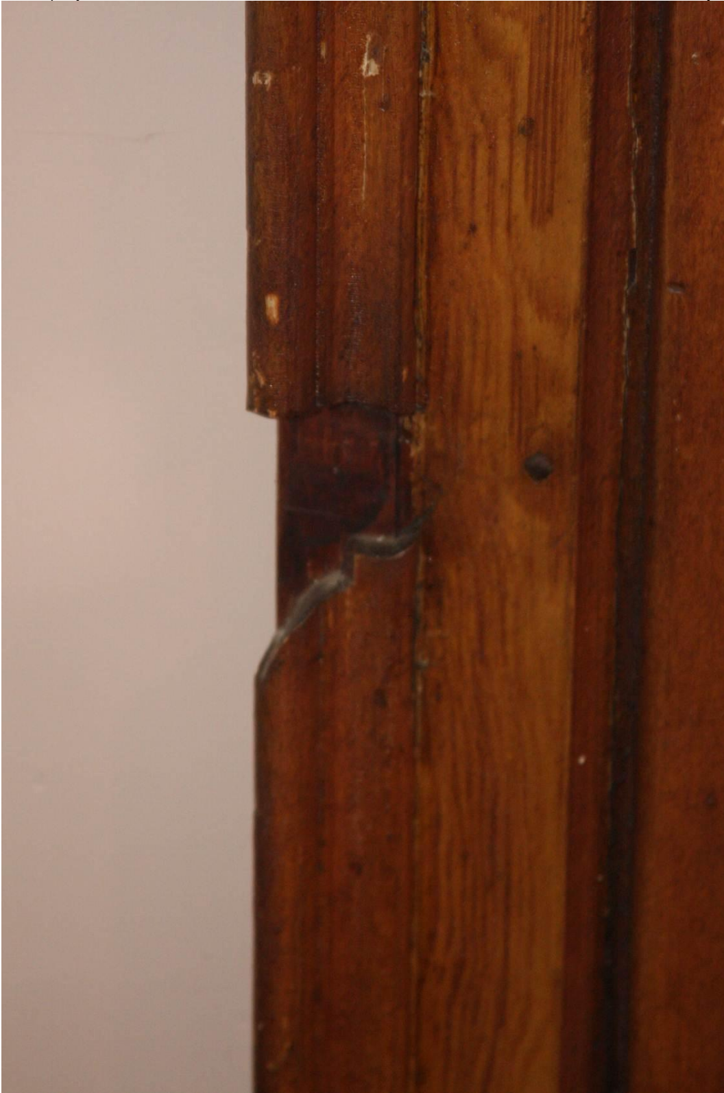
10 of 10 – Looking east at the front door surround at the point where the banking counter may have abutted the trim.
