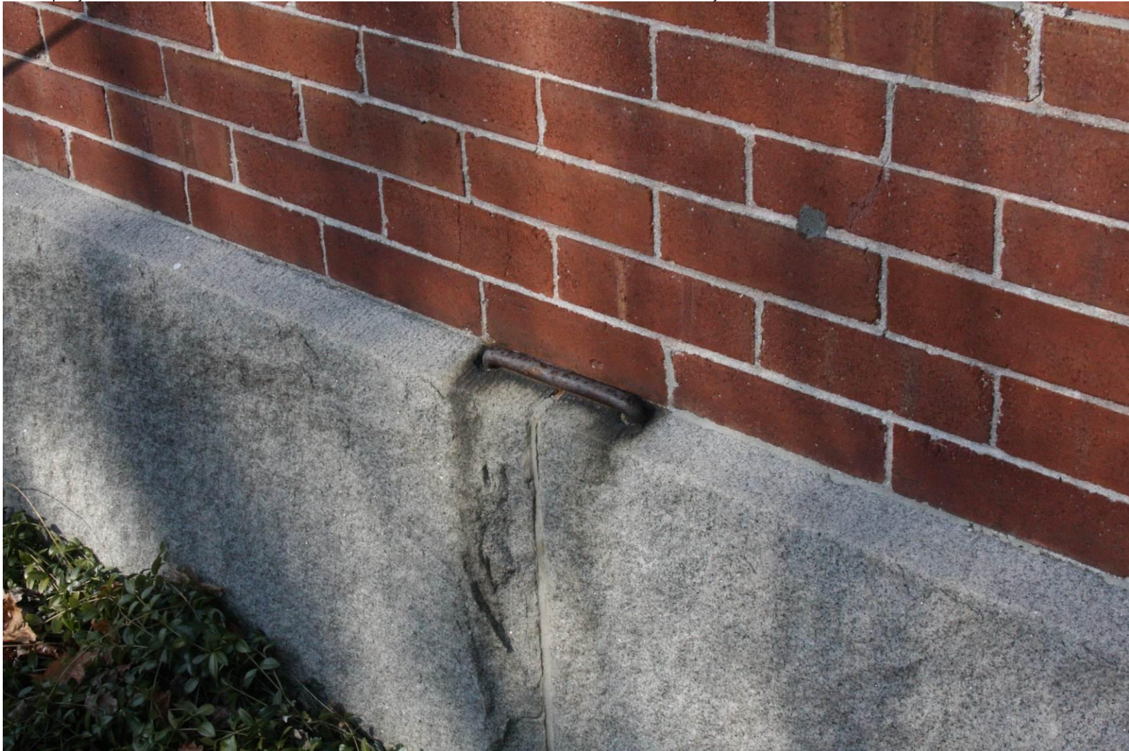
2 of 10 – Looking north at a detail of the south exterior wall and foundation.
