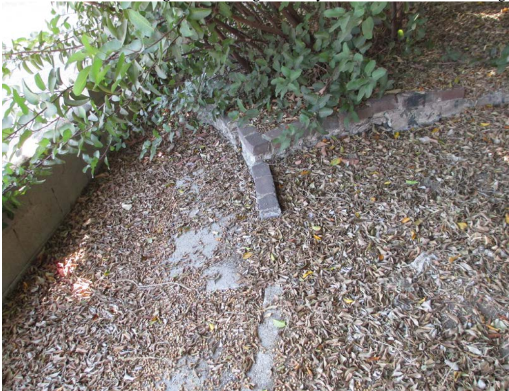
29 of 30. Exterior: Footing of one of original Hollywood School for Girls cottages
