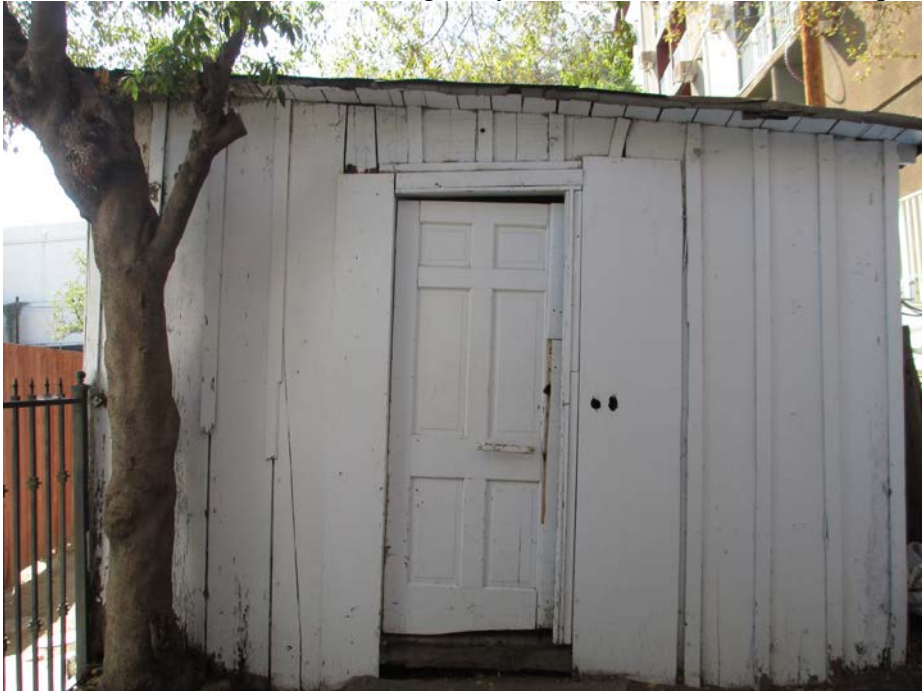
28 of 30. Exterior: Shed used originally as classroom and teachers' quarters, view west
