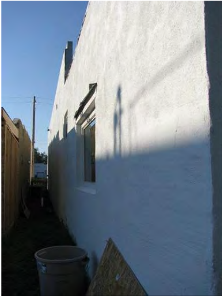
Description of Photograph: West Elevation, view to the South-southeast. Photo No. MT_CarterCounty_FirstNationalBankOfEkalakaAnd RickardHardwareStoreBuilding_0008
