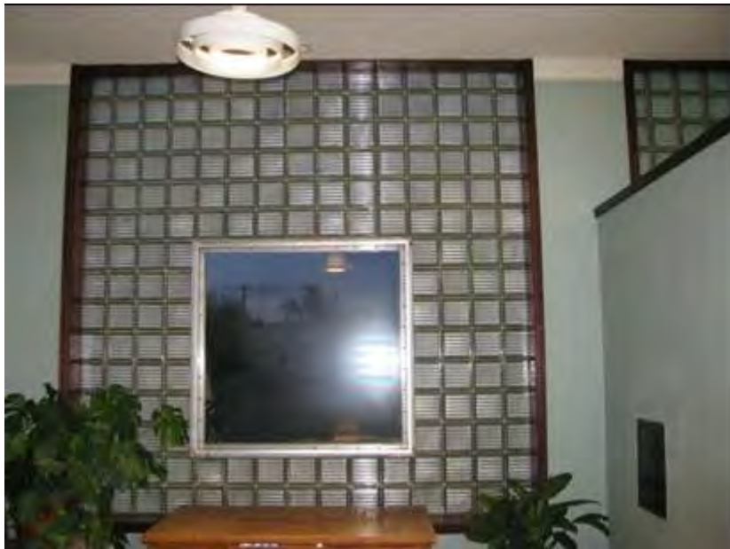
Description of Photograph: Close up of Interior of historic bank (now townhall) showing glass block window, view to the Southeast.
