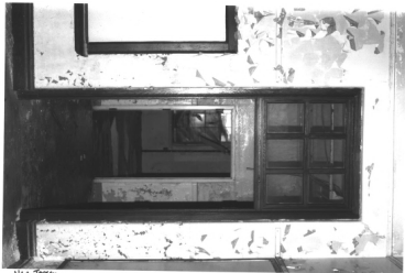
New Jersey Hudson County River Street School Photo # 7 of 9
