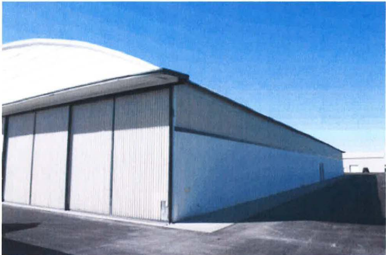
Figure 4. Falcon Field East Hangar, view of east-facing bay doors and north wall. Photo by Eric Vondy, State Historic Preservation Office, 2015.
