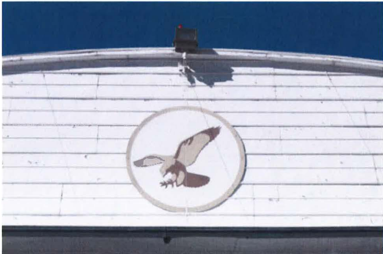
Figure 3. The Falcon emblem is mounted on the barrel gables over the bay doors on each hangar. The emblem and underlying galvanized tin sheathing are original material. Photo by Eric Vondy, State Historic Preservation Office, 2015.
