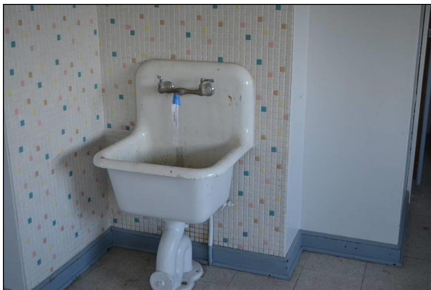
Photo #18 (WI_Eau Claire County_Eau Claire Vocational School_0018) Second floor room 205. Wash sink former kitchen area of vocational school.
