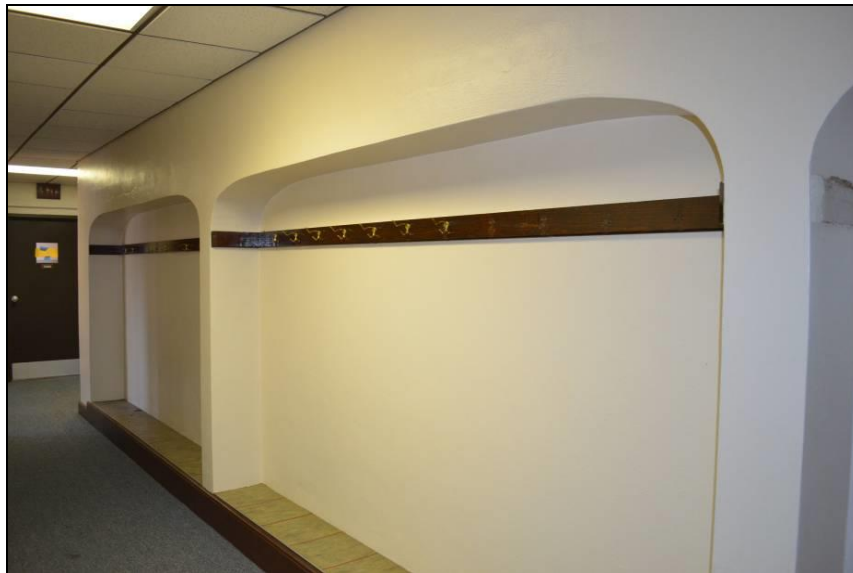
Photo #21 (WI_Eau Claire County_Eau Claire Vocational School_0021) Third floor corridor west wall. Coat hanger alcove of former vocational school.
