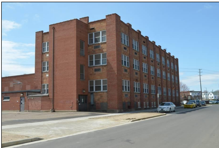
Photo #2 (WI_Eau Claire County_Eau Claire Vocational School_0002) East façade (right) and south elevation (left), camera facing northwest.
