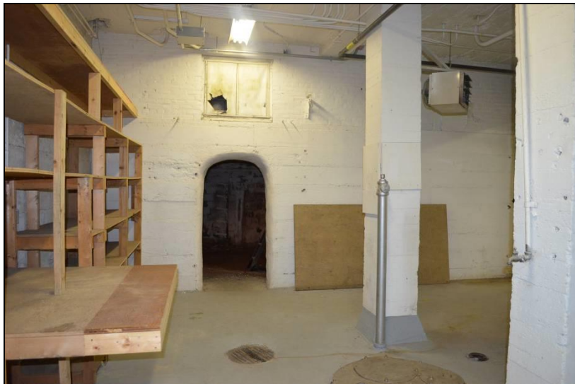
Photo #25 (WI_Eau Claire County_Eau Claire Vocational School_0025) Lower level, storage LL-B. Looking west.at entrance to fuel room from former boiler room of vocational school.
