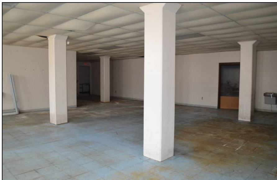
Photo #23 (WI_Eau Claire County Eau Claire Vocational School_0023) Lower level, room LL3. Looking southwest. Machine shop area of former vocational school.
