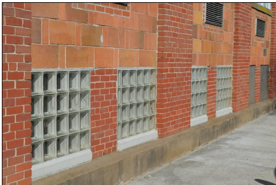
Photo #15 (WI_Eau Claire County_Eau Claire Vocational School_0015) Detail glass block windows and concrete plinth foundation.
