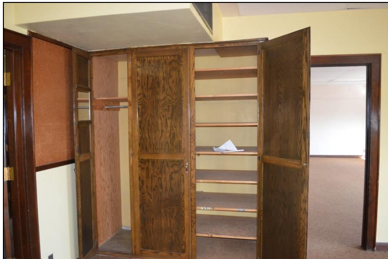
Photo #19 (WI_Eau Claire County_Eau Claire Vocational School_0019) Third floor room 307, northwest corner. Built in closet area of former vocational school.
