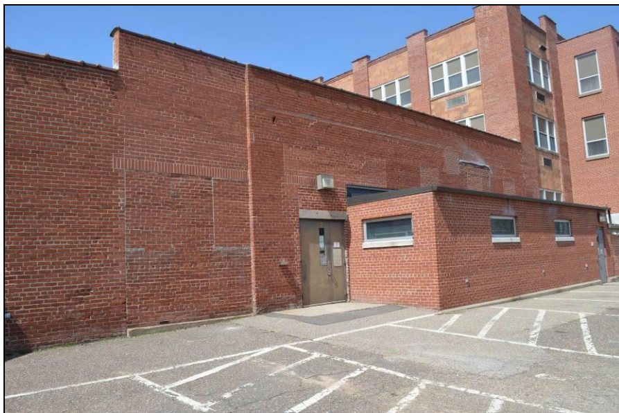
Photo #12 (WI_Eau Claire County_Eau Claire Vocational School_0012) South façade, bricked in areas, camera facing northeast.
