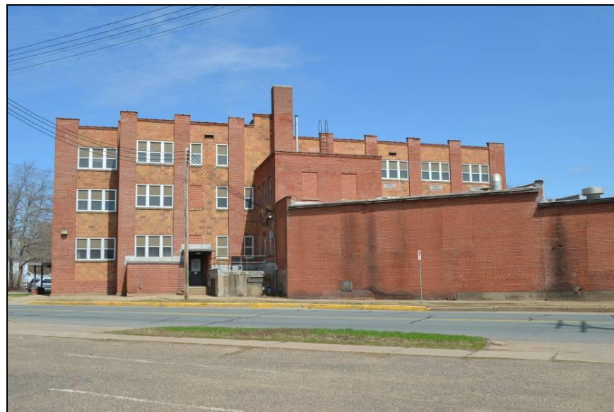
Photo #6 (WI_Eau Claire County_Eau Claire Vocational School_0006) West façade, camera facing east.
