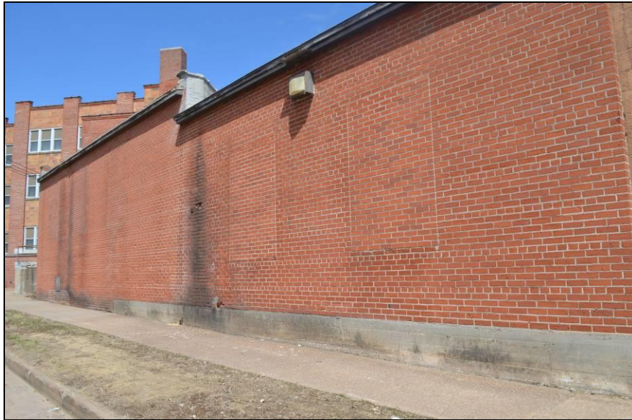
Photo #11 (WI_Eau Claire County_Eau Claire Vocational School_0011) West façade, bricked in windows, camera facing northeast.
