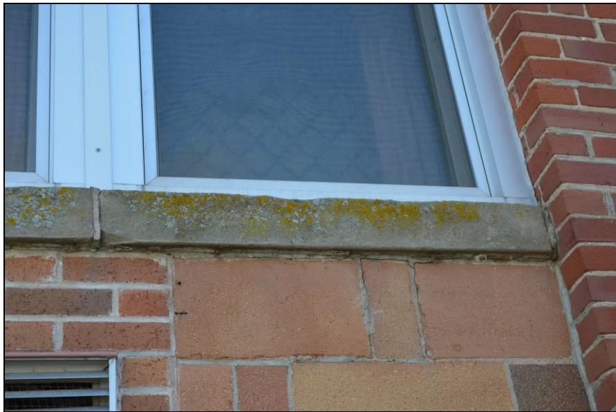
Photo #13 (WI_Eau Claire County_Eau Claire Vocational School_0013) Detail of window, stone sill, common bond brick pattern, and buff tile exterior.
