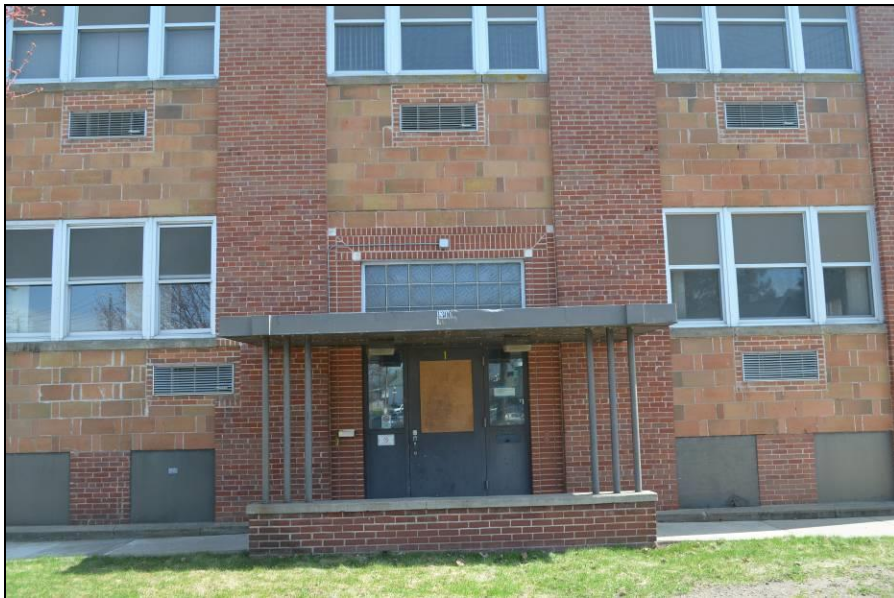
Photo #9 (WI_Eau Claire County_Eau Claire Vocational School_0009) North façade, front door, camera facing south.
