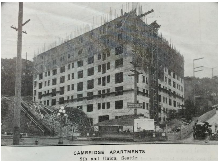
The Cambridge under construction, Cover Photo, Pacific Builder & Engineer , Volume 28, #43, "Build Reinforced Concrete Structures," 1922.
