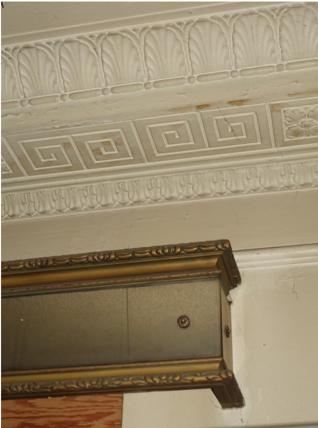
0018. Interior, detail view of Lobby ceiling & window valance (in office, above acoustic ceiling).
