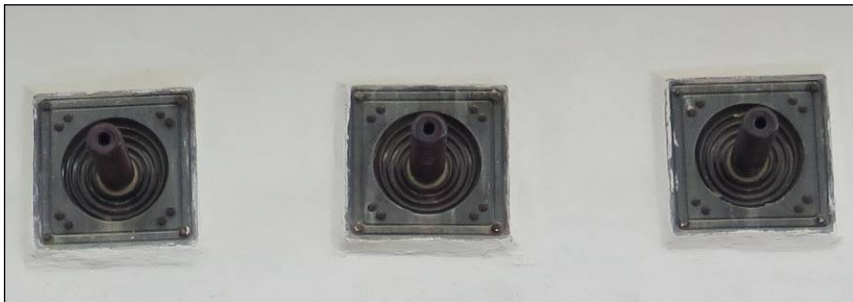
Close-up view of the insulators that extend through the south wall of the substation section of the Center Point Depot looking North at the exterior.
