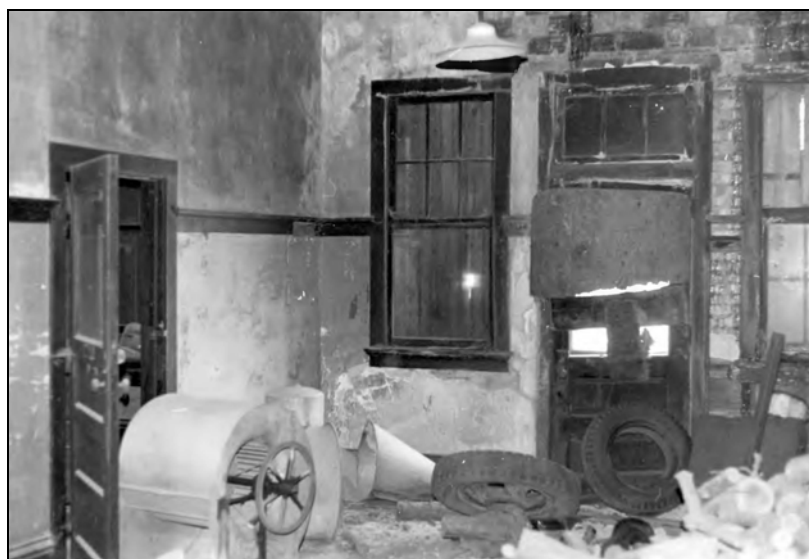
Interior of WCF&N Center Point Depot and Substation in the 1980s prior to first rehabilitation. Photographs on file State Historical Society of Iowa, Center Point Depot files, Des Moines, Iowa.
