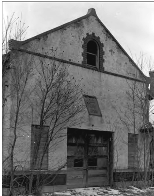
Gable-end of WCF&N Center Point Depot and Substation in the 1980s prior to first rehabilitation. Window panes in the gable-end are missing as are some of the panes in the freight doors, with the flanking windows boarded over.
