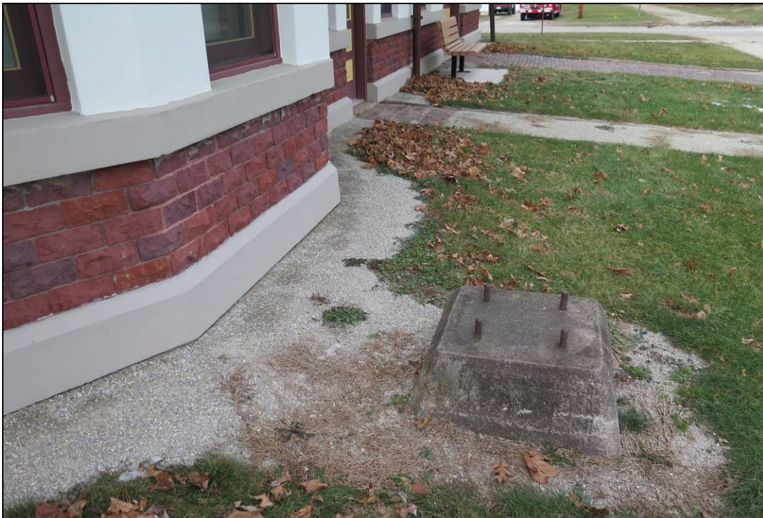
Photograph of the east side of the Center Point Depot showing the square concrete base where the signal post was once attached and some of the brick-paved brick sidewalks between the depot and the former interurban grade.
