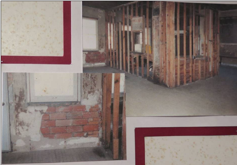
Photographs taken during the 1980s rehabilitation showing the damaged plaster removed from the interior of the ticket office and waiting room area of the Center Point Depot. Copy obtained from the Center Point Historical Society Collections, Depot Museum, Center Point, Iowa.
