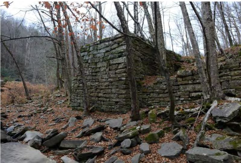
Photo 18: WV_RaleighCounty_BeckleyMillSite_0018 Looking west at the east wall of the bridge abutment where it joins the south end of the east wall of the Beckley Mill foundation.
