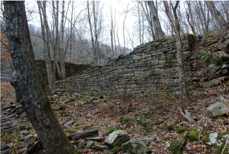
Photo 17: WV_RaleighCounty_BeckleyMillSite_0017 Looking west at the east wall of the Beckley Mill foundation and the wheel well.
