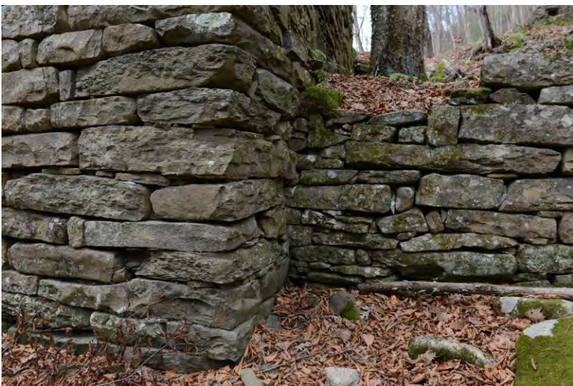
Photo 4: WV_RaleighCounty_BeckleyMillSite_0004 Mill foundation where it is overlapped by the bridge abutment, view facing west.
