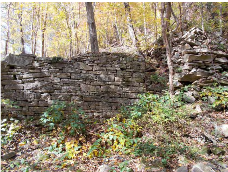
Photo 6: WV_RaleighCounty_BeckleyMillSite_0006 Loose masonry on north side of wheel well (at right of view), view facing northwest.
