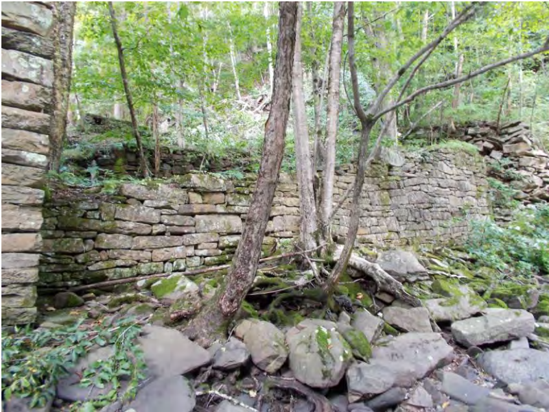
Photo 1: WV_RaleighCounty_BeckleyMillSite_0001 Beckley Mill foundation, east or front wall facing creek, view facing west.
