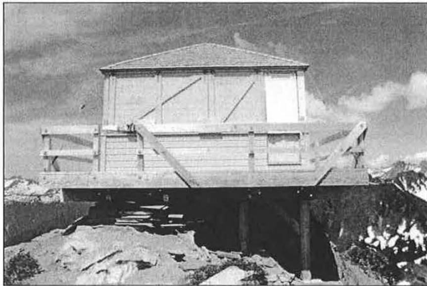
Figure 5. Green Mountain Lookout south elevation, in its current condition, after substructure and catwalk were replaced (stairway not completed), also freshly painted, July 2010. (Gary Paull, Forest Service photograph).
