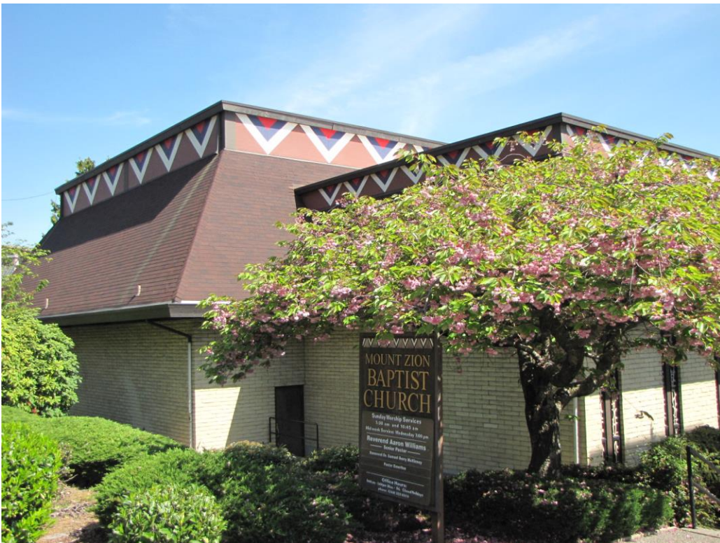
3 of 20 Mt. Zion Baptist Church detail of exterior roof and wall configuration.
