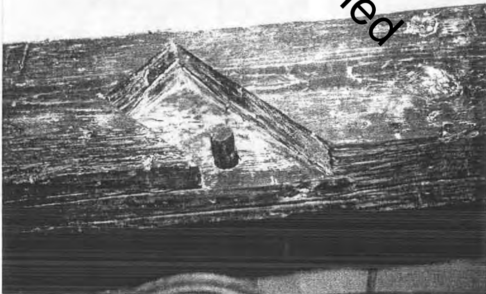
Figure 12: Vacant mortise for half-dovetail joint on south (side) girt
