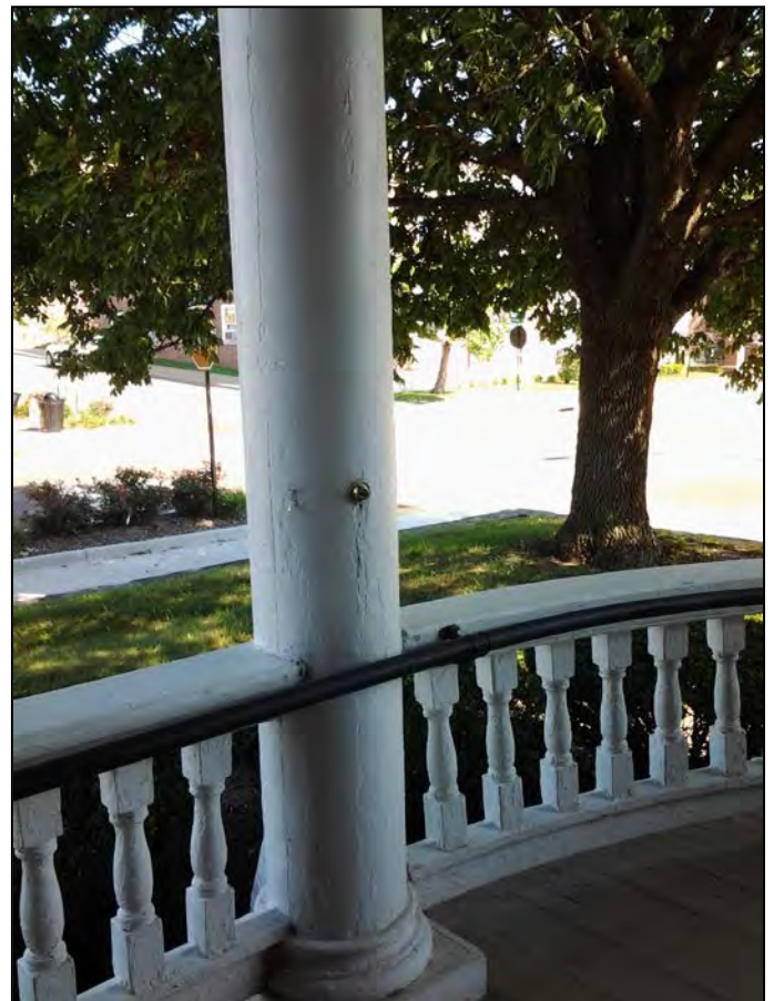
Figure F11. Front porch column with buzzer button for calling attendant – no longer functional. Camera pointed southeast.
