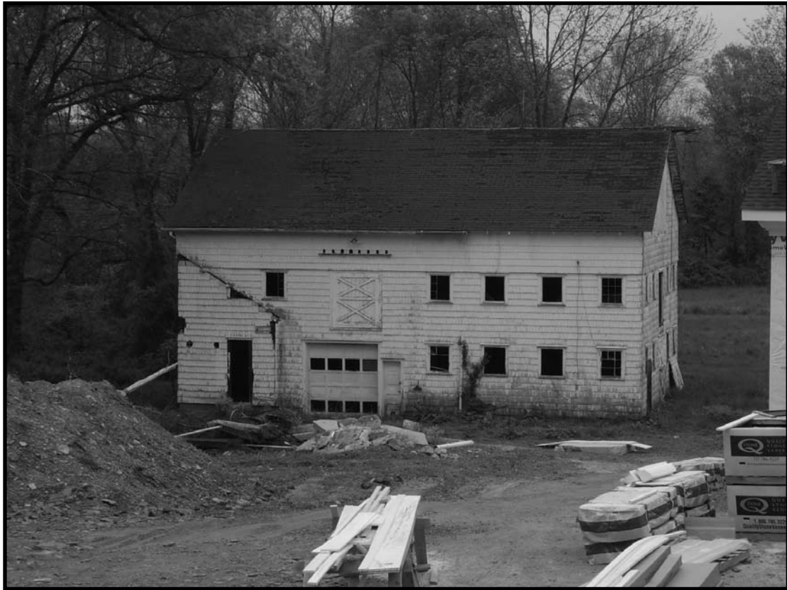
Princeton Nurseries Historic District, Plainsboro and South Brunswick Townships, Middlesex County, New Jersey
