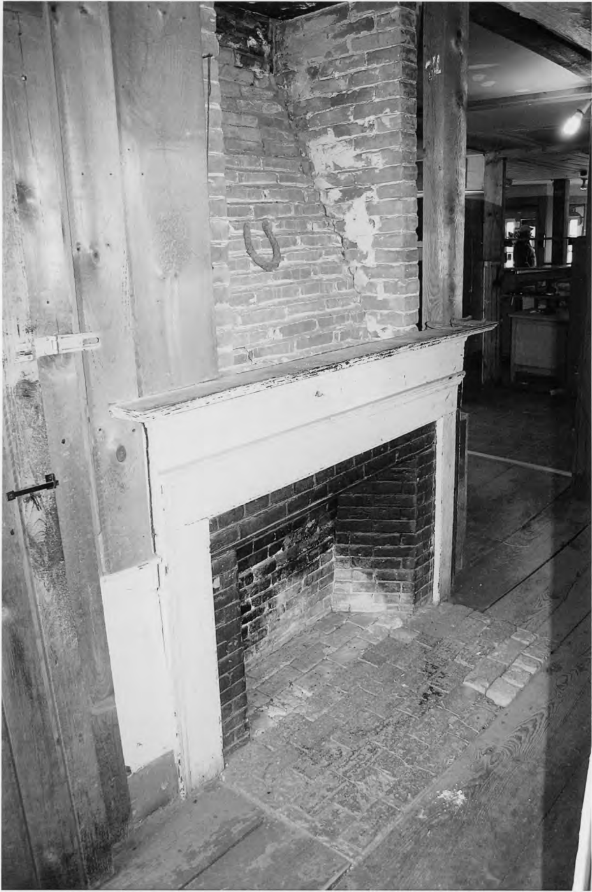
Broad Brook House; Guilford, Windham Co., VT (11/1/2010 by L. Papazian, Digital images are on file at the Vermont Division for Historic Preservation) Photo. # 8 of 10: Detail of Federal fireplace surround and wainscot
