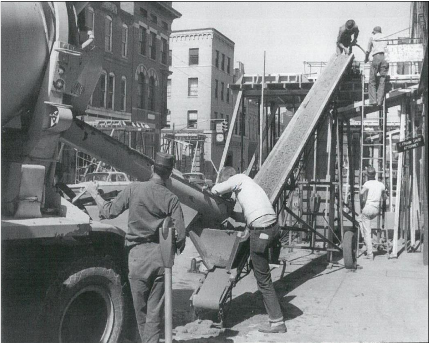
Figure 15. Construction of support columns for the Skymart, circa 1965. View from 200 block of West Main Street. City National Bank Building (#50) and Hamilton Bank Building (#49) are visible in the background.
