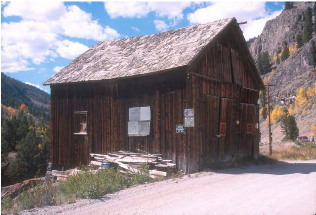
HP 21. 2001 photo of the southeastern and northeastern sides of Building 36, looking west. This building collapsed and was removed soon thereafter.
