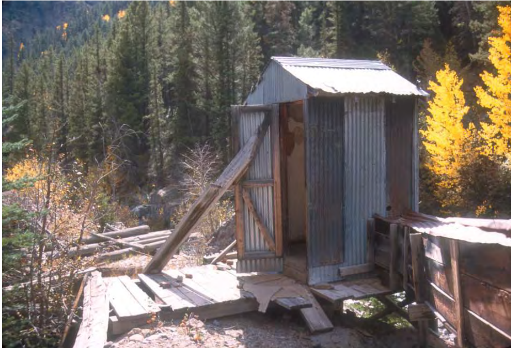
HP 12. 2001 photo of the small corrugated sheet metal shed (Building 13) with wooden boardwalk in front and water pipe in covered box to right. View is to the south. This building is now laying on its front side.
