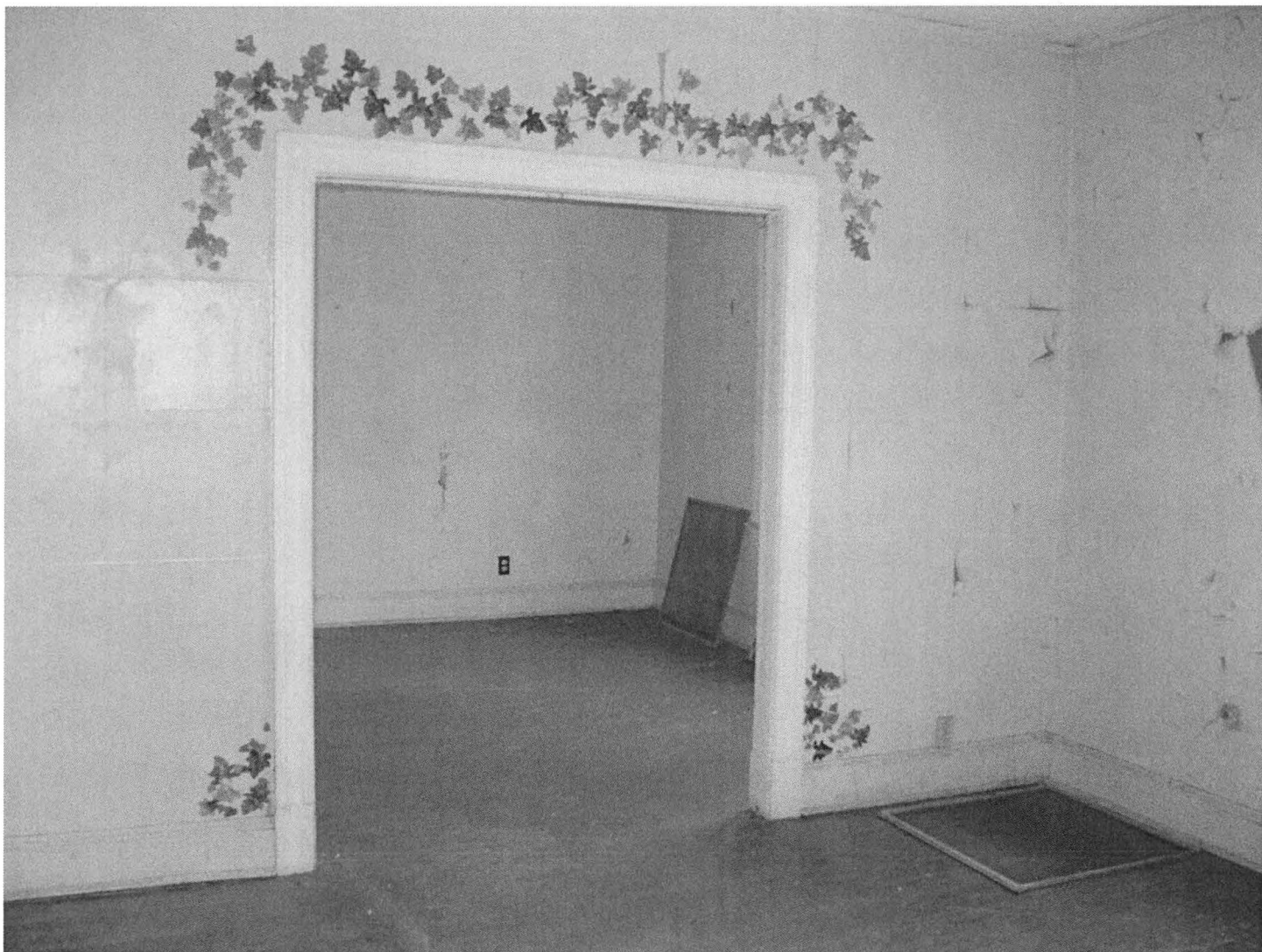
Interior of apartment, showing typical floor, wall, and trim details. Camera facing southeast. Photograph 10 of 11
