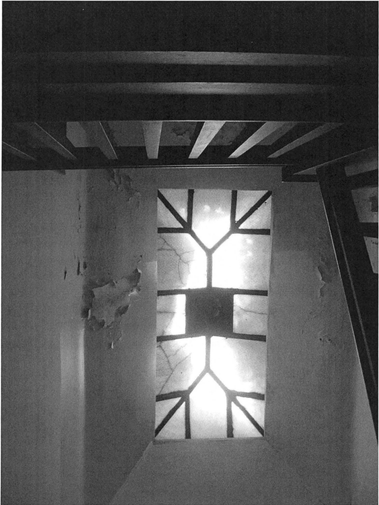
Interior of eastern entry stairwell, showing light shaft details. Camera facing up, with east being at the top of the image. Photograph 8 of 11
