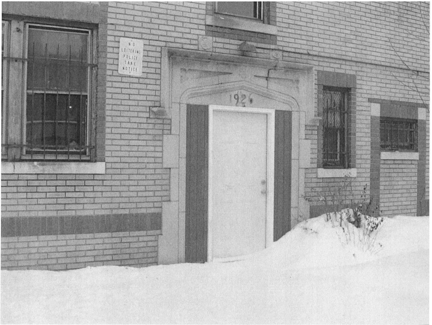
South (side) elevation of building from Ashley Street, showing south entry detail. Camera facing northeast. Photograph 3 of 11
