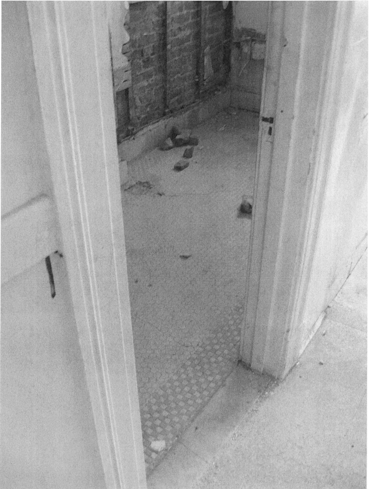
Interior of apartment, showing typical bathroom details. Camera facing northwest. Photograph 11 of 11
