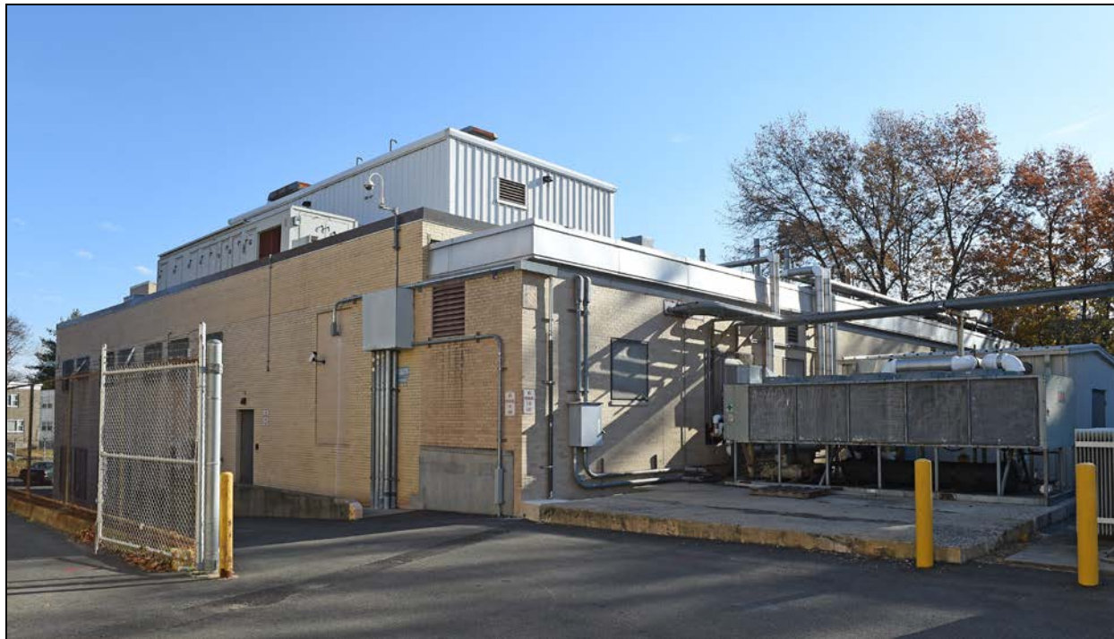
Figure 11. (above) Perspective view of Building #7 and view showing mechanical equipment to the southwest, November 2017 (VA).
