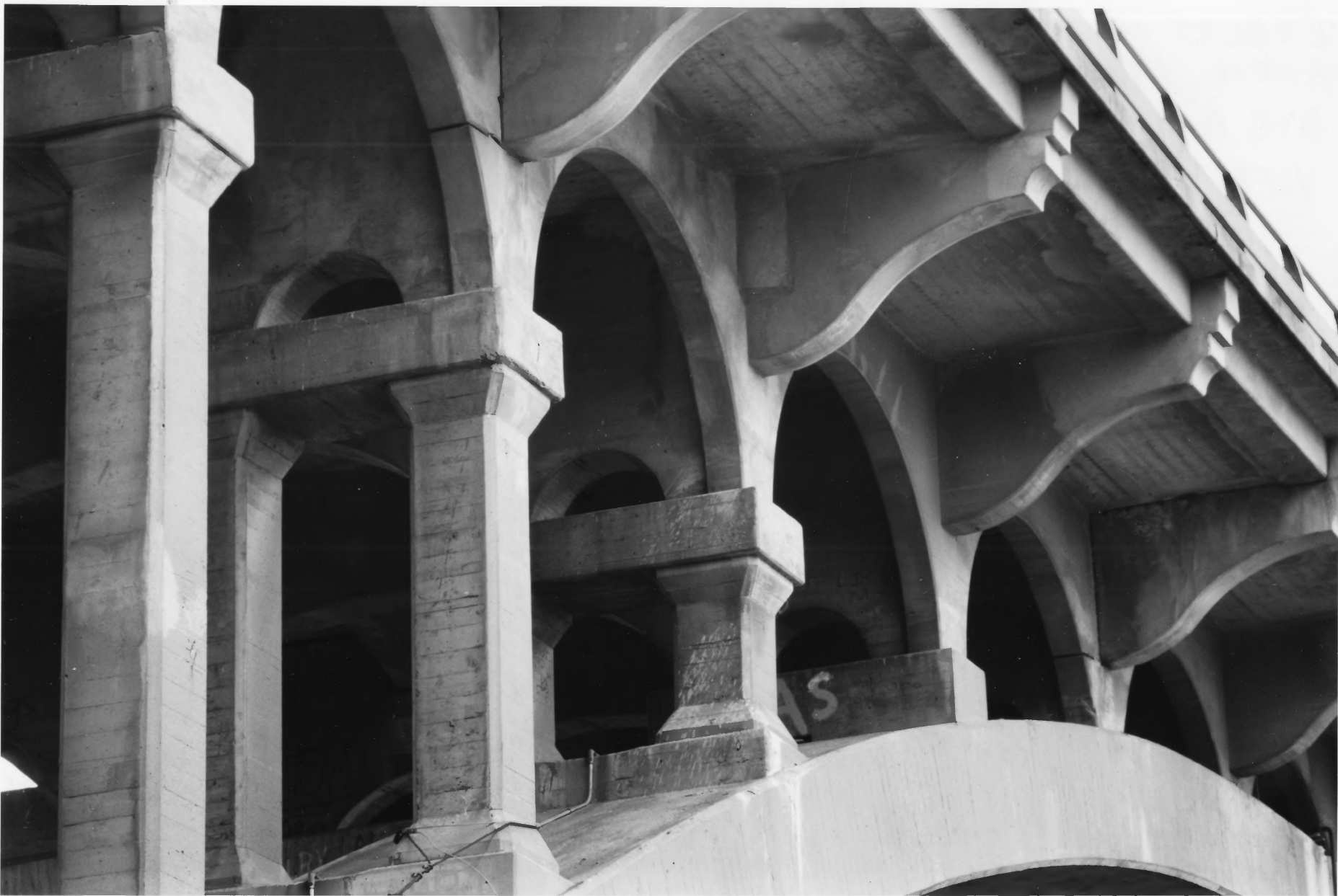
INTERCITY / FORD BRIDGE NO. 3575 ST. PAUL, RAMSEY CO., MN PHOTO I.D. 09727# 17A
