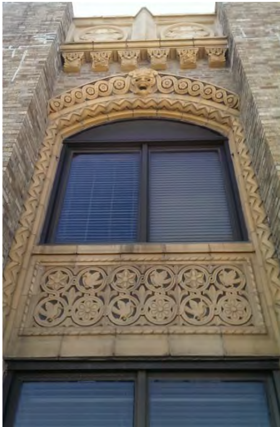
Photo 19: Exterior view of typical terra cotta and masonry detailing Camera facing west Date: 2015
