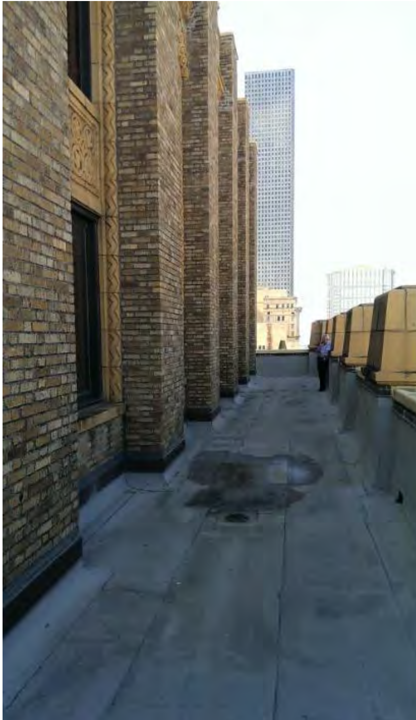
Photo 15: Exterior view of typical window and bulkhead at stepped roof areas levels 17, 19, and 21 Camera facing northeast Date: 2015
