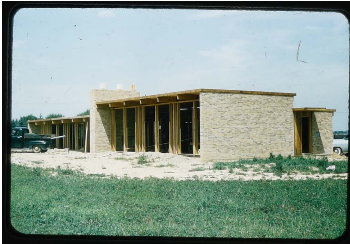
FIGURE 12: Lavin House, south and east elevations during construction, before brick was painted, 1955. Source: Wisconsin Historical Society Archives.
