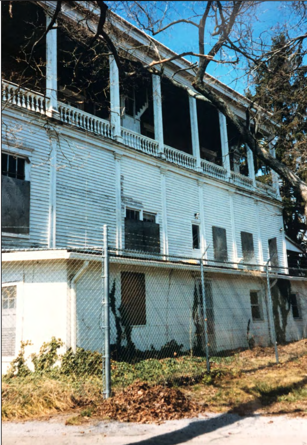
Figure 42: Rear (East) Elevation of Clover Bottom Mansion in 1990 showing the changes that had occurred during the State Era. Photo from the Clover Bottom File, Tennessee Historical Commission.
