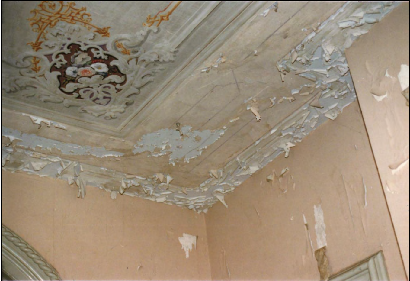
Figure 44: Deteriorated Ceiling in the Parlor, including stenciling, 1990. Photo in Clover Bottom File, Tennessee Historical Commission.
