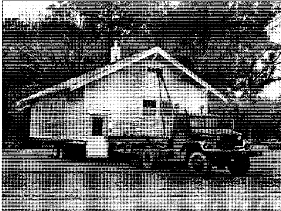
Figure 9: Original site, house turned and ready to move, view northwest (photo by Linda McCann, 2006)
