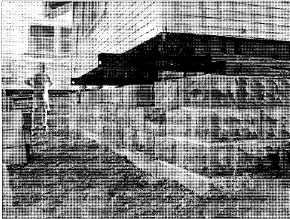
Figure 11: Garage in place above new foundation, view southwest (photo by Linda McCann, 2006)
