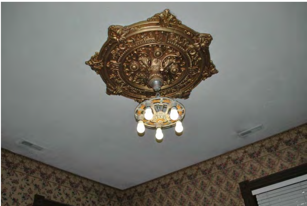
Photograph 9 of 9 Main floor, interior, parlor, plaster ceiling medallion detail. Camera facing southwest.
