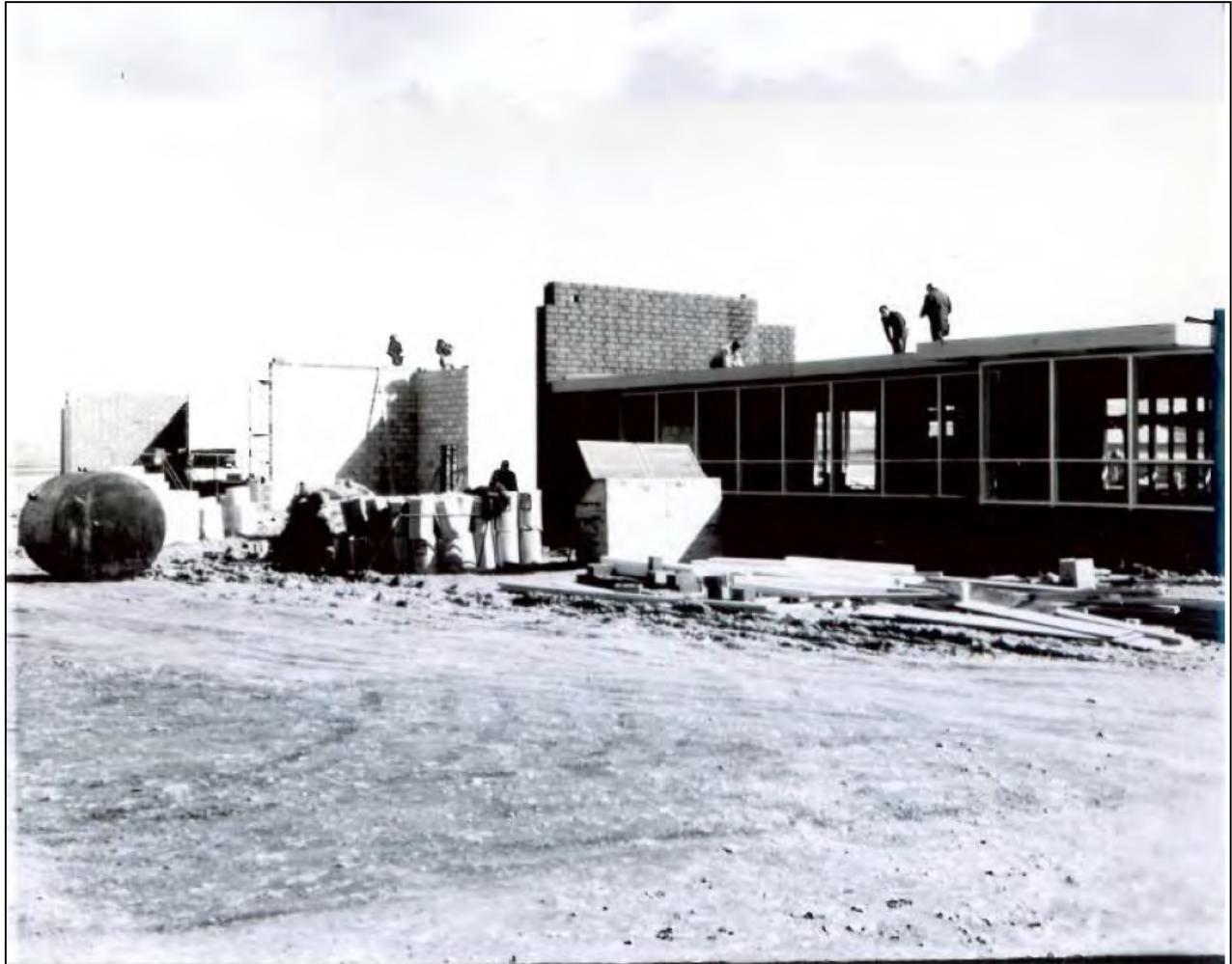
The Montana Aeronautics Commission Operations Building under construction, 1958. North façade. View to the southeast.
