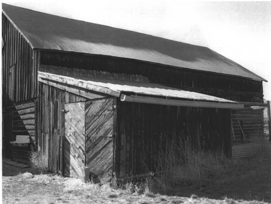
Wold Barn #10. South and east elevations, shed-roof addition to east elevation, view to the northwest.
