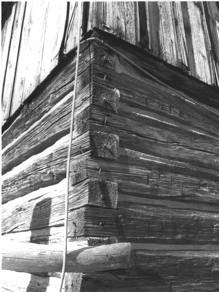
Wold Barn #16. Notching detail southwest corner of log addition, view to the northeast.
