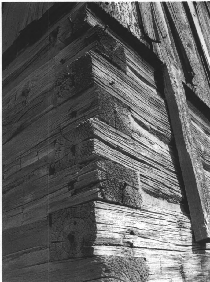
Wold Barn #15. Notching detail, northwest corner of main component, view to the southeast.
