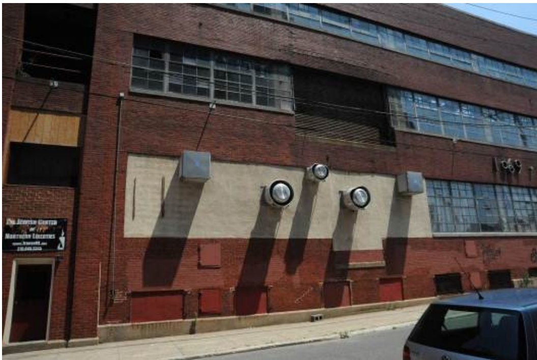
Figure 6: Ortlieb's Bottling House, west and south elevations before rehabilitation. Photos: Emily T. Cooperman, 2013.
