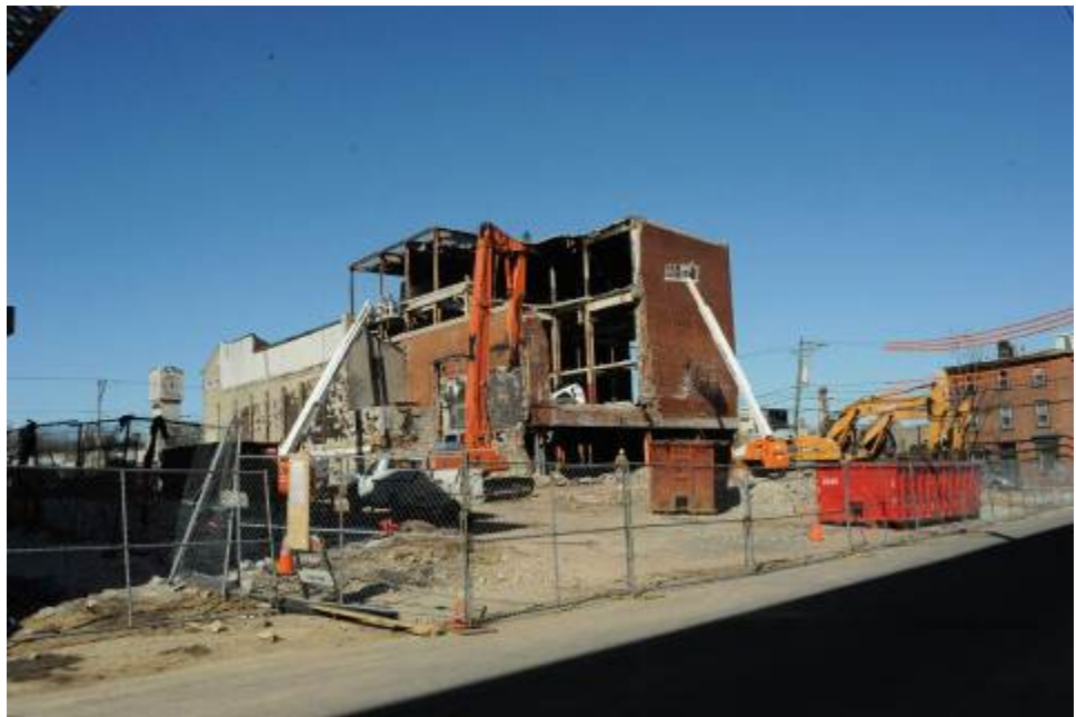
Figure 5: Ortlieb's western buildings being demolished, February, 2014. Top: looking west from the intersection of N. American and Poplar Streets; Bottom: looking northwest from N. American Street. Photos: Emily T. Cooperman
