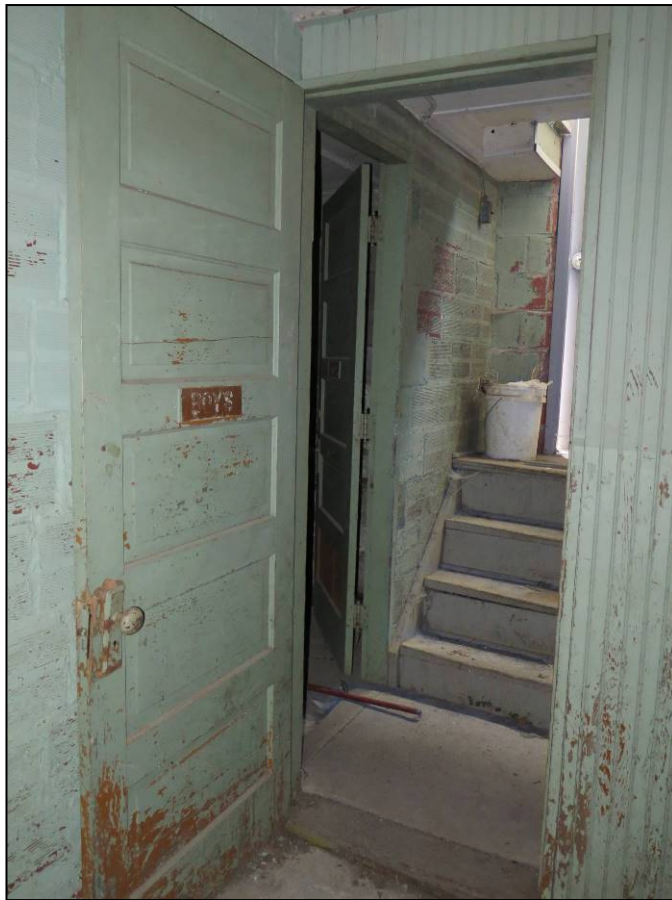
Figure 19. Door to east-side rest room labeled “BOYS” looking SSE towards stairs to outside entry door landing. Photograph taken by Leah Rogers, Tallgrass Archaeology LLC, October 9, 2017
