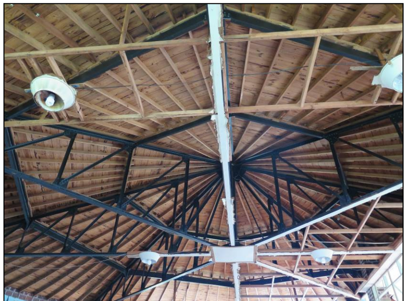
Figure 6. Steel truss system for the gymnasium roof. Photograph taken by Leah Rogers, Tallgrass Archaeology LLC, October 9, 2017.
