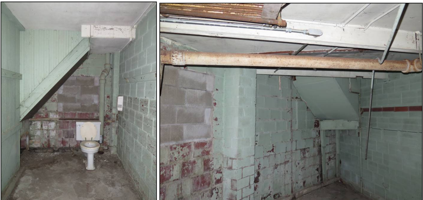
Figure 18. Basement rooms in Yale High School Gymnasium, with the boys' rest room to left looking south and the girls' locker room to right looking NW.
