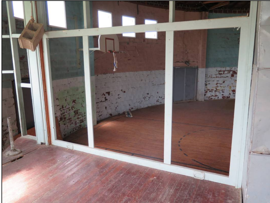
Figure 10. Side panels that lift-up using a pulley system on either side of the stage looking NW from the stage. Photograph taken by Leah Rogers, Tallgrass Archaeology LLC, October 9, 2017.
