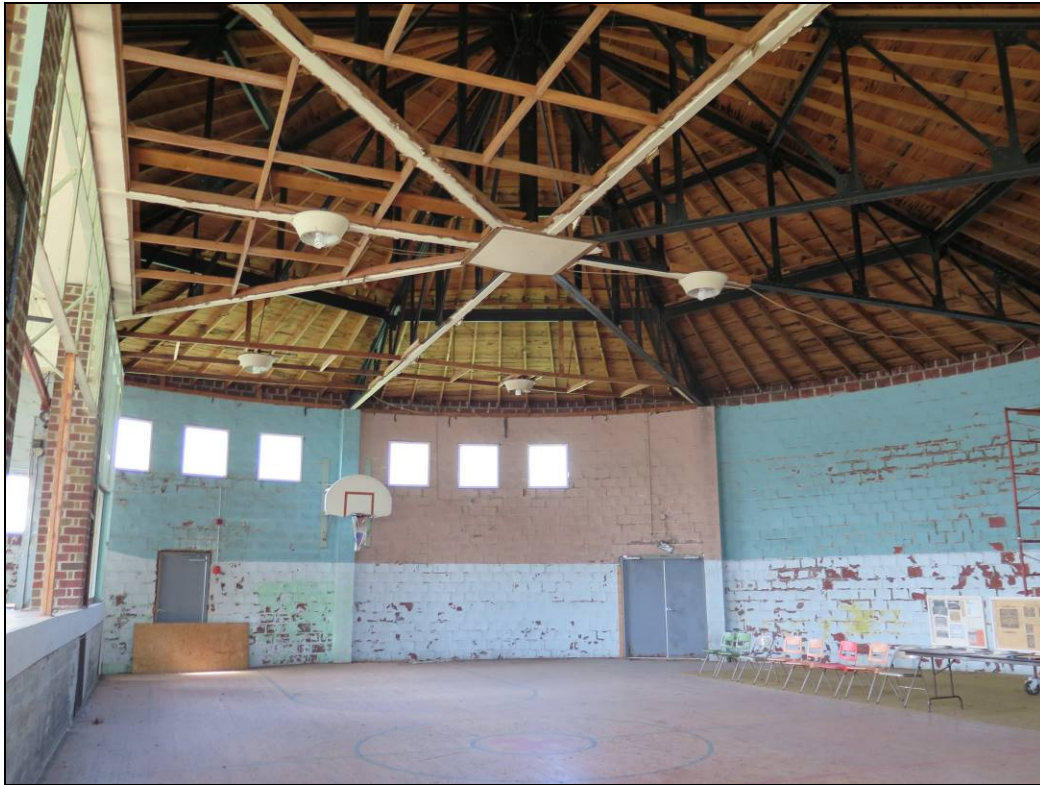
Figure 7. Interior of Yale High School Gymnasium showing roof truss system above the basketball court looking west. The elevated stage is to the left side of this view, with the area of the former bleachers to the right. Photograph taken by Leah Rogers, Tallgrass Archaeology LLC, October 9, 2017.
