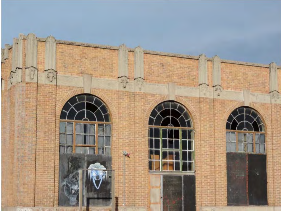
Photograph 5 of 13 Detail of south facade over the main entry. Camera facing northeast.
